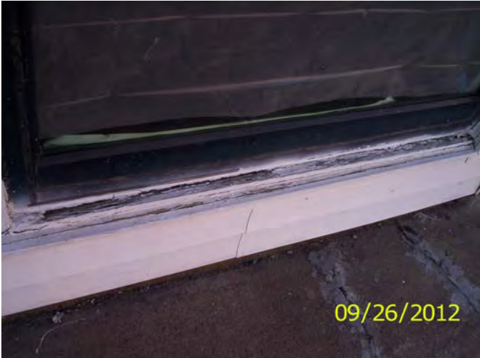
Damaged window opening
