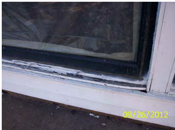
Damaged window opening
