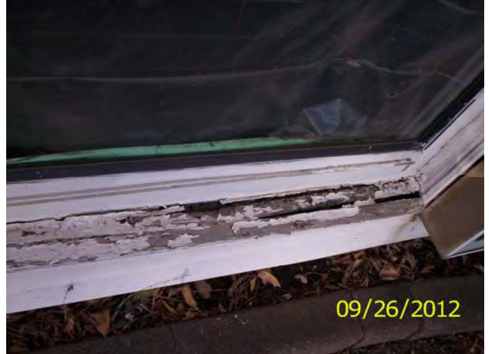
Damaged window opening
