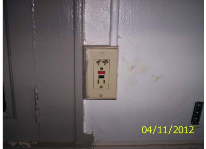
Fire damaged electrical outlet in common bathroom
