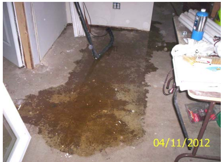
Standing water on the basement floor
