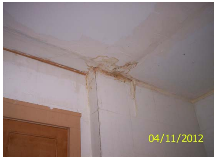
Water damaged ceiling and wall
