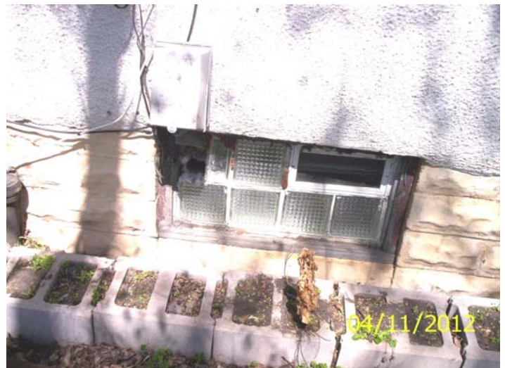
Damaged, open dry vent
