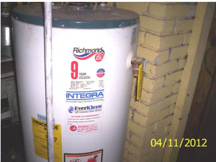
Water heater missing overflow tube
