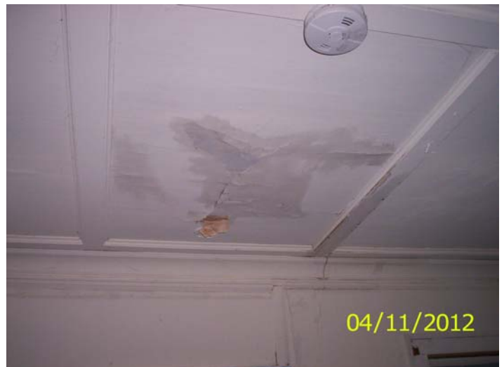
Water damaged ceiling
