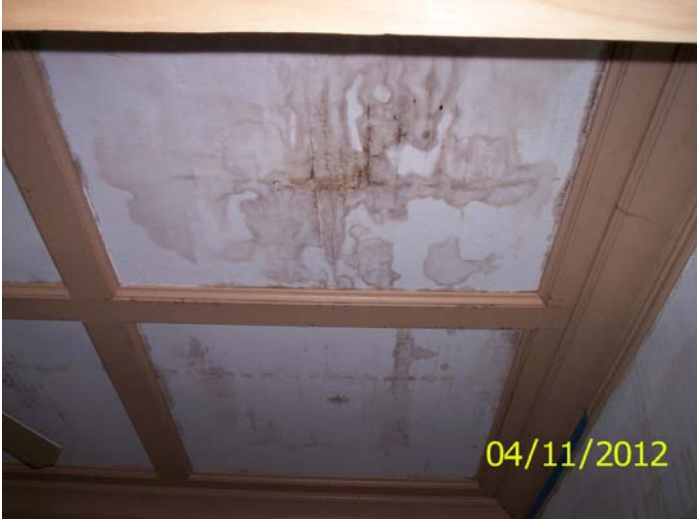
Water damaged ceiling
