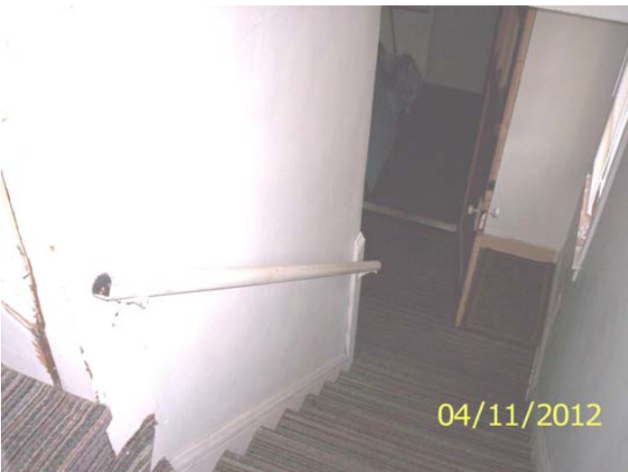
Unapproved hand rail
