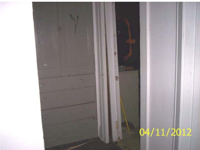
Damaged door frame
