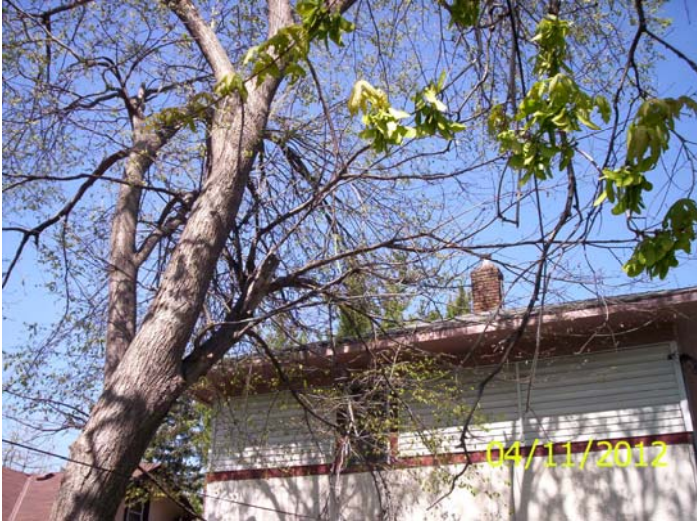
Roof damage from tree
