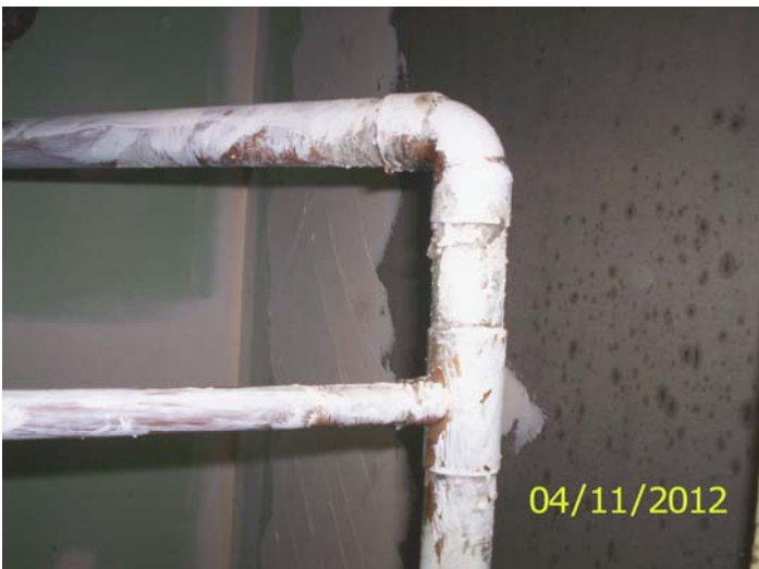
Upper pipe joint leaking, mold on wall
