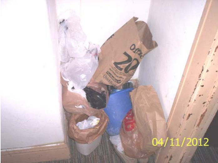
Refuse and debris
