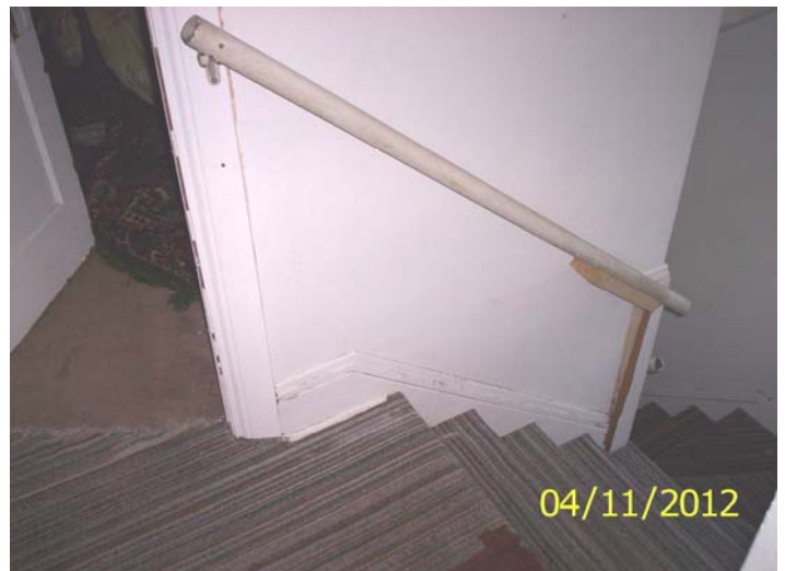
Unapproved hand rail
