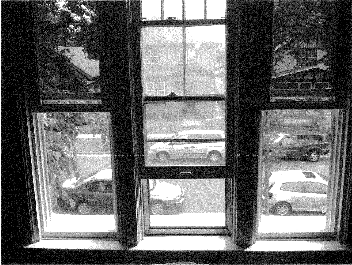
Attachment 1: Center window is existing and conforming. Side windows are replacement inserts of the same type proposed for the center window.
