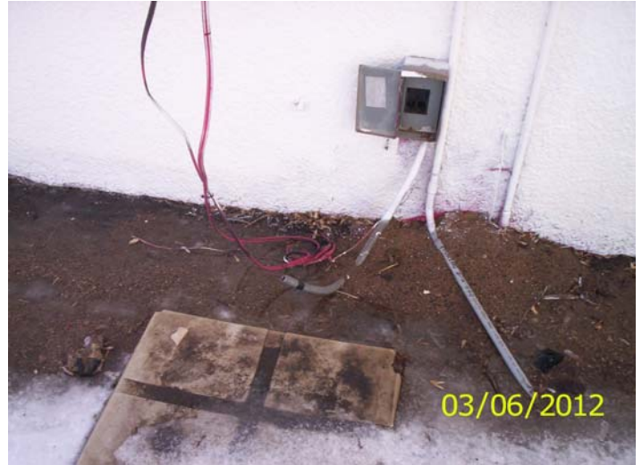
Damaged components of the central air conditioner
