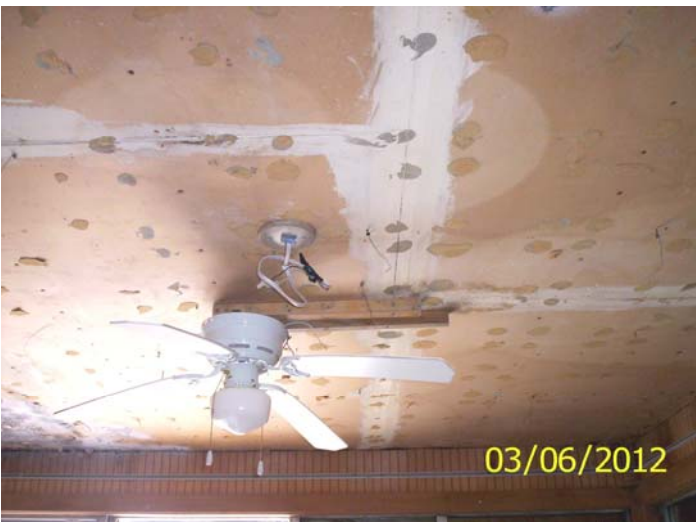
Open wiring, no fixture box
