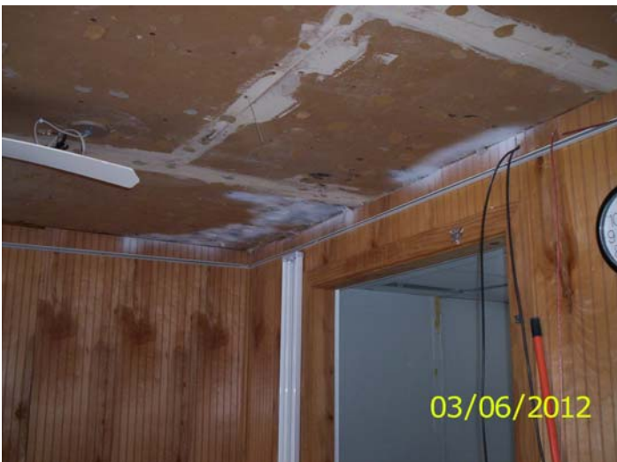
Mold on ceiling
