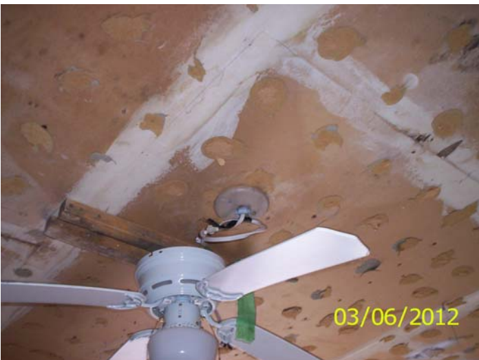
Open wiring, no fixture box
