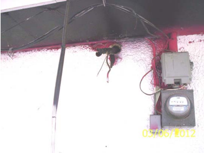
Damaged components of the central air conditioner
