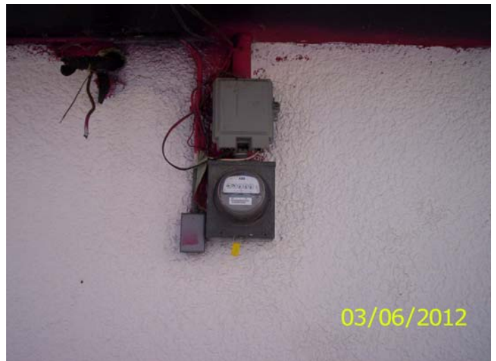
Electric meter yellow tagged off
