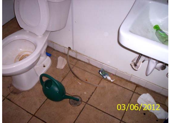
Dry toilet trap, staining in front of toilet
