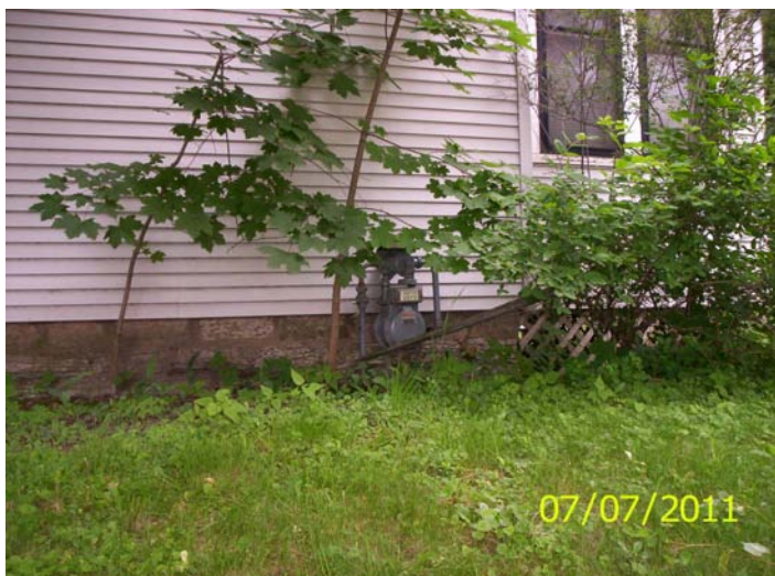
Gas meter locked off
