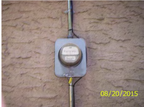
Electric meter yellow tagged off
