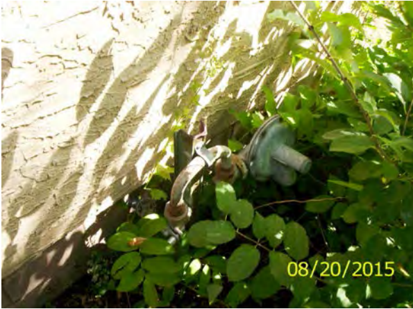
Locked gas meter
