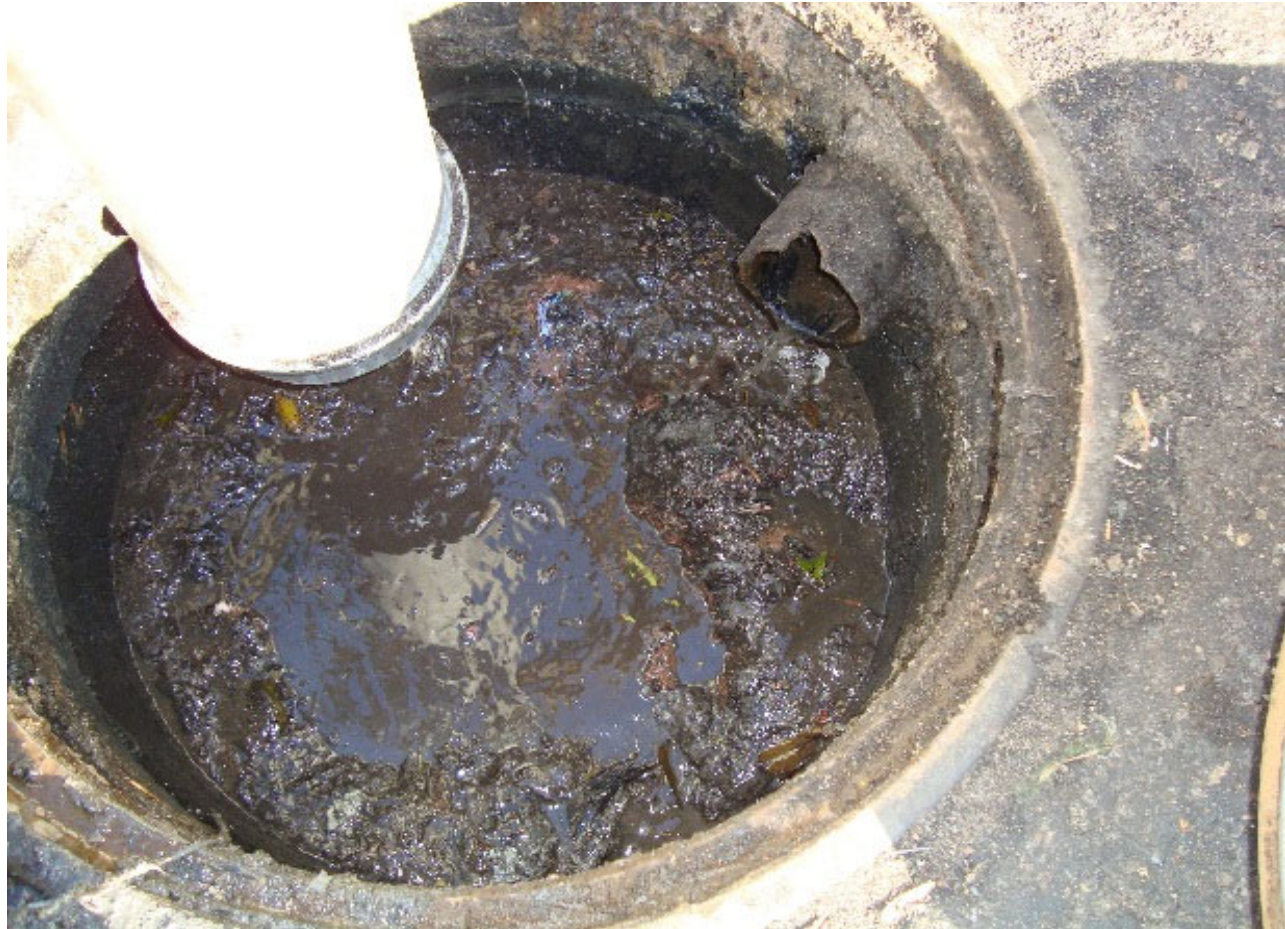
Sanitary Discharge, Private Storm Drain
