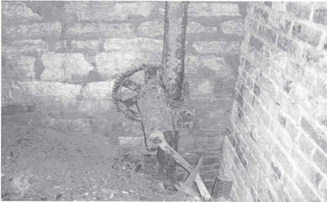
Image 19: (North Section) Existing mechanical in northwest corner.
