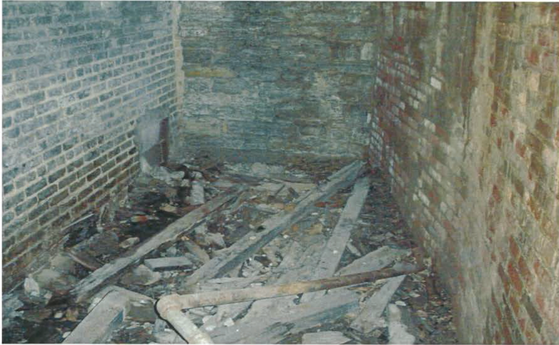
Image 15: (South Section) Debris on floor.
