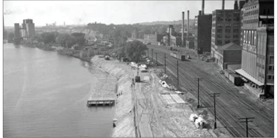
Figure 37. Filling along the future Shepard Road below the West Publishing Co. and Northern States Power and other plants, ca. 1947.
