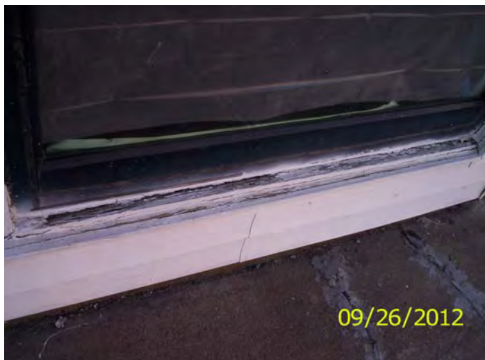
Damaged window opening
