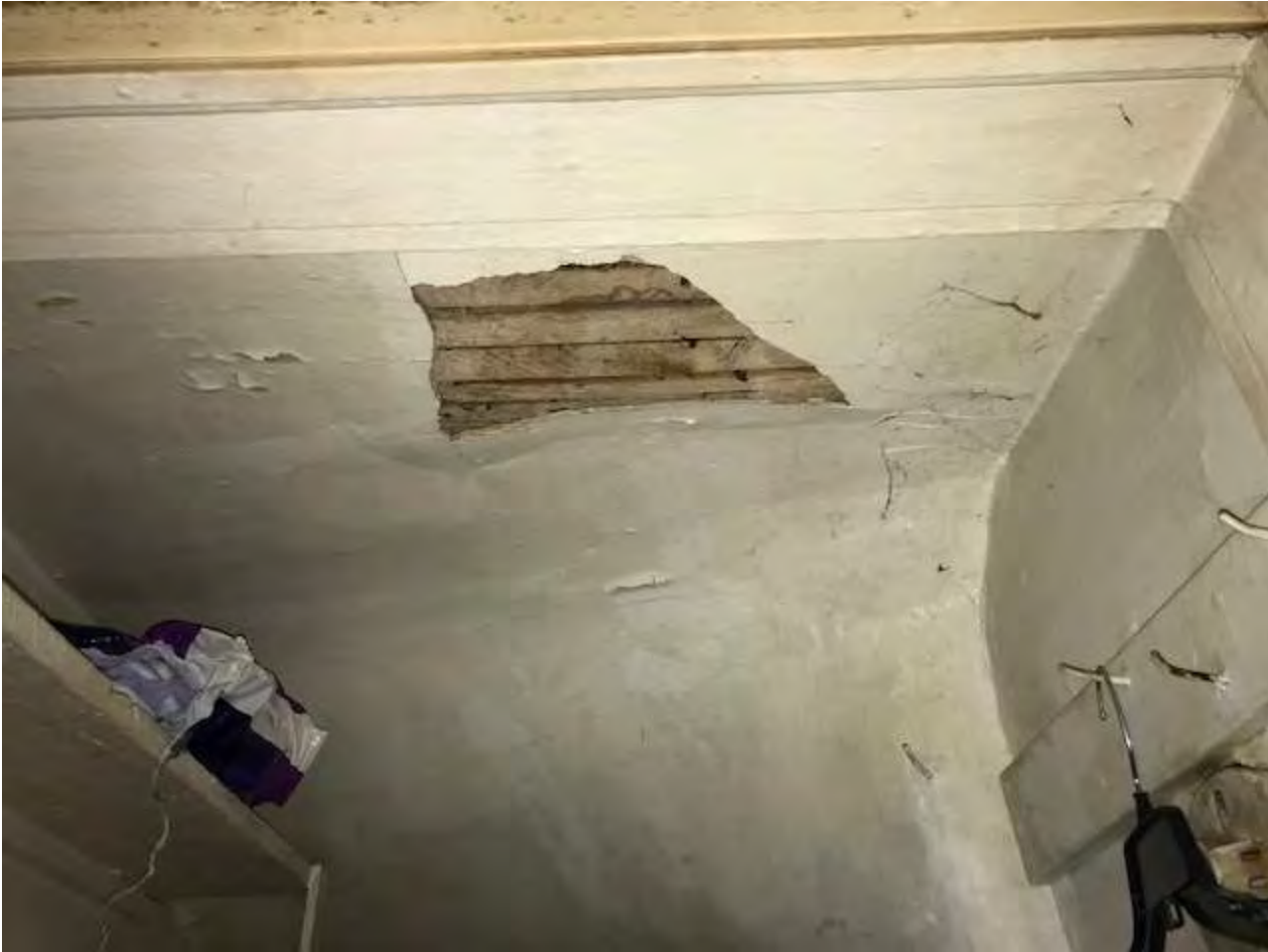
Ceiling above entryway to basement, Unit 1
