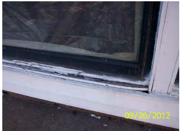
Damaged window opening
