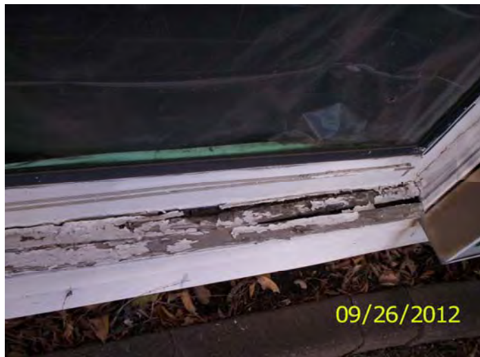
Damaged window opening
