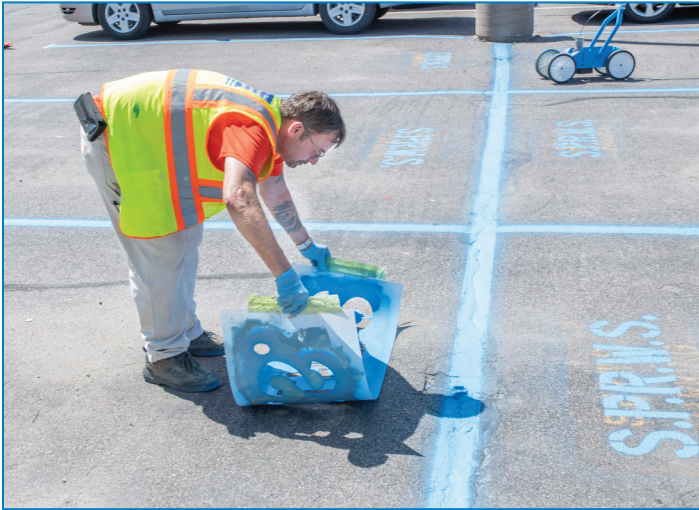
Jerry Pierce, painter, lays down the stencil to paint the designated parking areas for SPRWS vehicles last month. These spots are reserved for SPRWS vehicles and should not be used by staff for their personal use.
