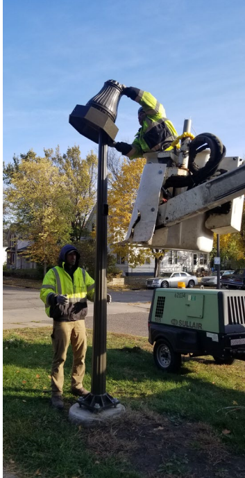
Lighting at Roy Wilkins Park
