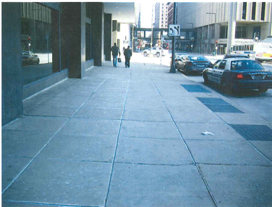
Photo 2: 18 feet wide, North side of 5 th St between Cedar St and Minnesota St
