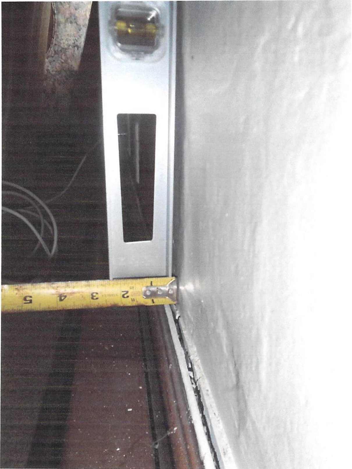
Photo 11: Inside face of interior wall behind the brick façade along the north wall was out of plumb a little less than \frac{1}{4} " in 4ft.
