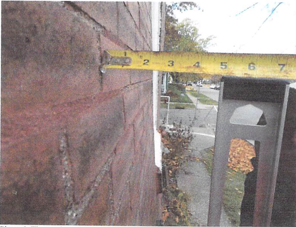
Photo 6: The north wall west of the window opening was approximately 4-3/4" out of plumb in 4ft.
