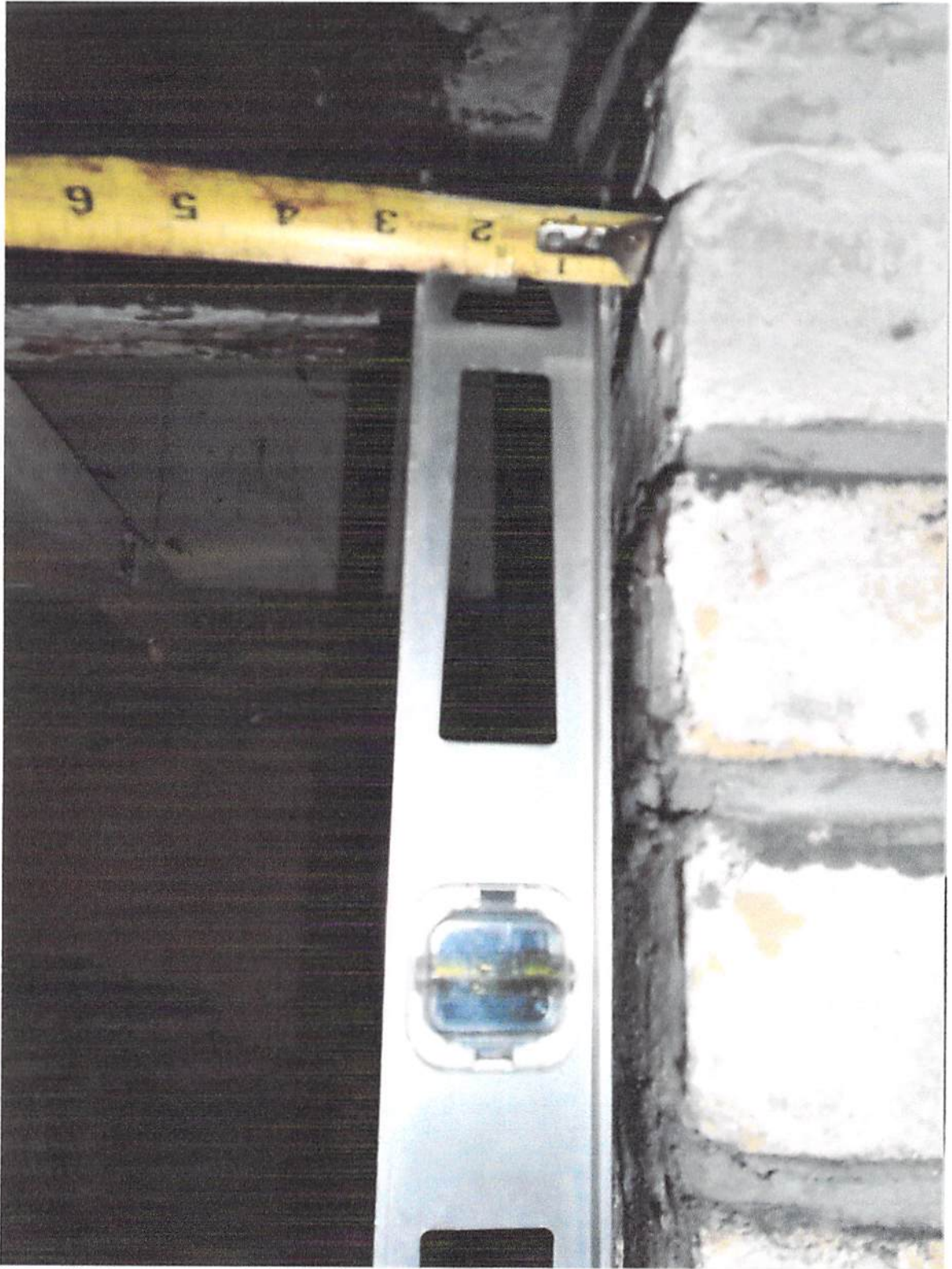
Photo 10: Measurement of the plumbness of the foundation wall west of the basement window on the north side of the residence.
