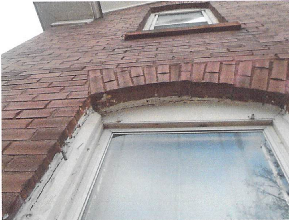
Photo 4: Deteriorated sealant observed around jamb and window head or easternmost window.
