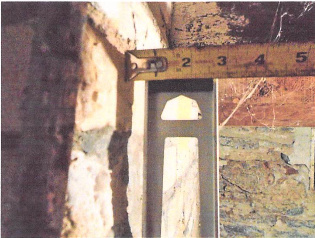
Photo 9: Measurement of the plumbness of the foundation wall east of the basement window on the north side of the residence.
