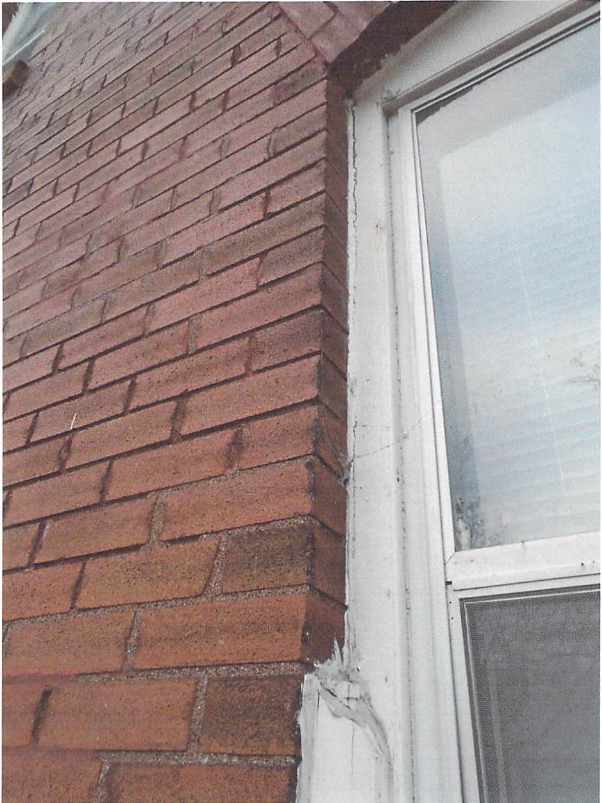
Photo 3: Deteriorated sealant on wood molding around perimeter of window stops show of window head.
