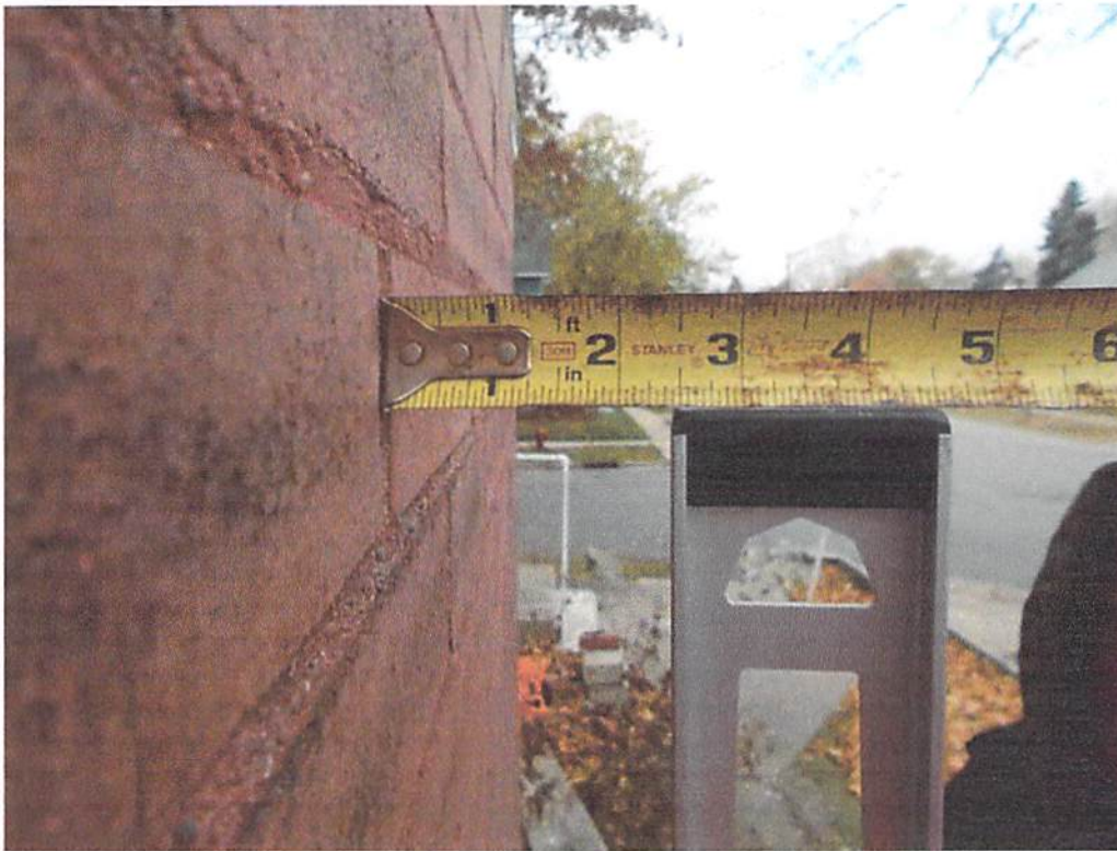
Photo 8: The north wall west of the window opening was approximately 2.5" out of plumb in 4ft.
