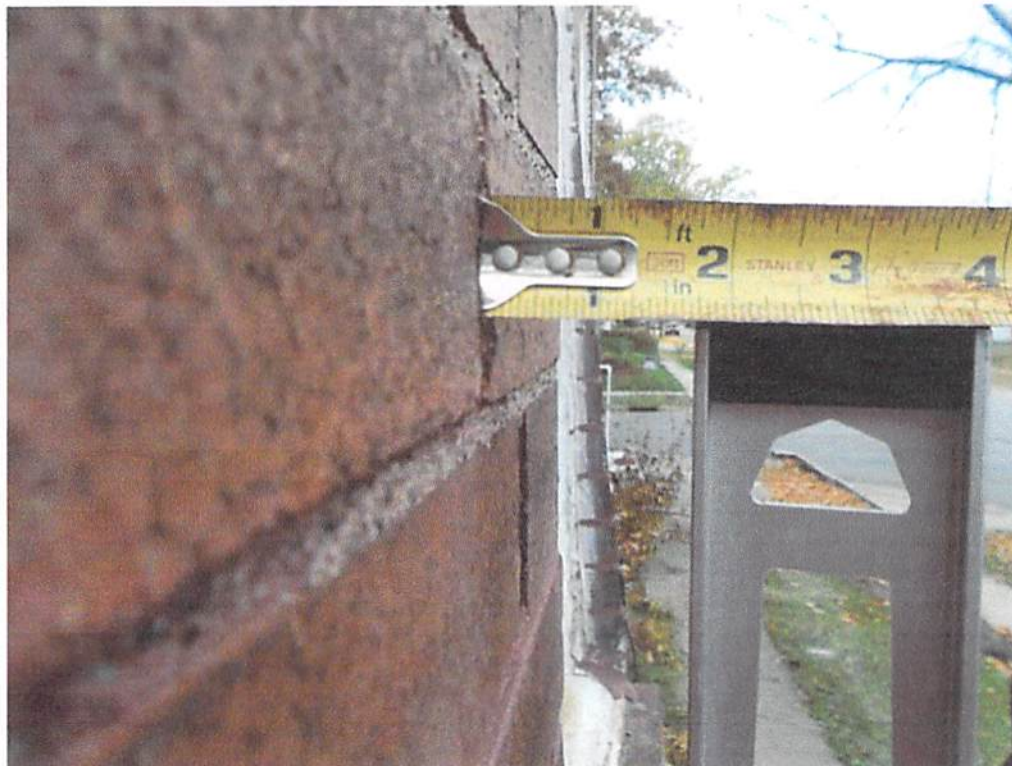
Photo 5: The north wall east of the window opening was approximately 1-3/4" out of plumb in 4ft.
