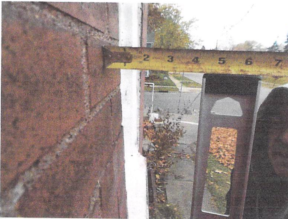
Photo 7: The north wall east of the window opening was approximately 4-3/16" out of plumb in 4ft.
