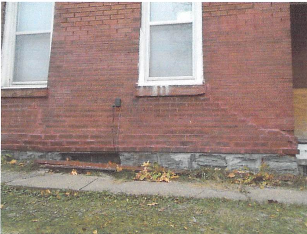
Photo 2: Another photo of the north wall in question, with stair step cracking starting at the sill of from the westernmost window.
