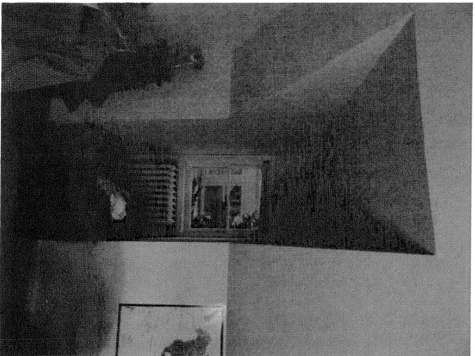
Existing 3 rd floor Unit 4 bedroom escape window
