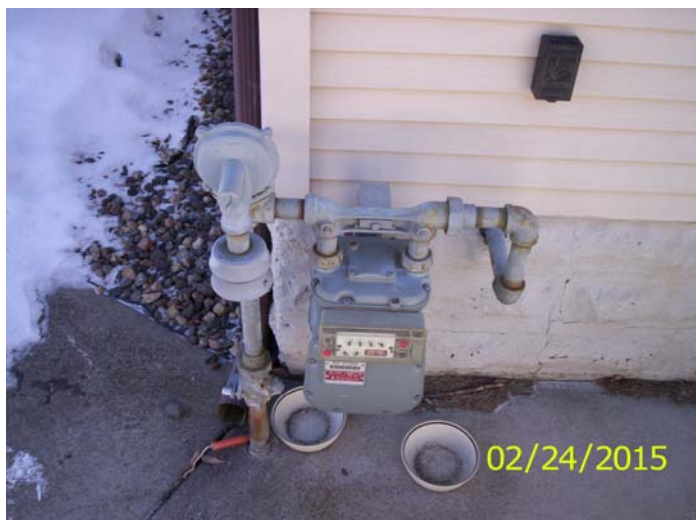
Locked gas meter
