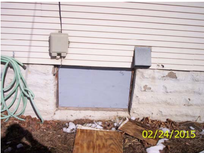
Boarded south side basement window
