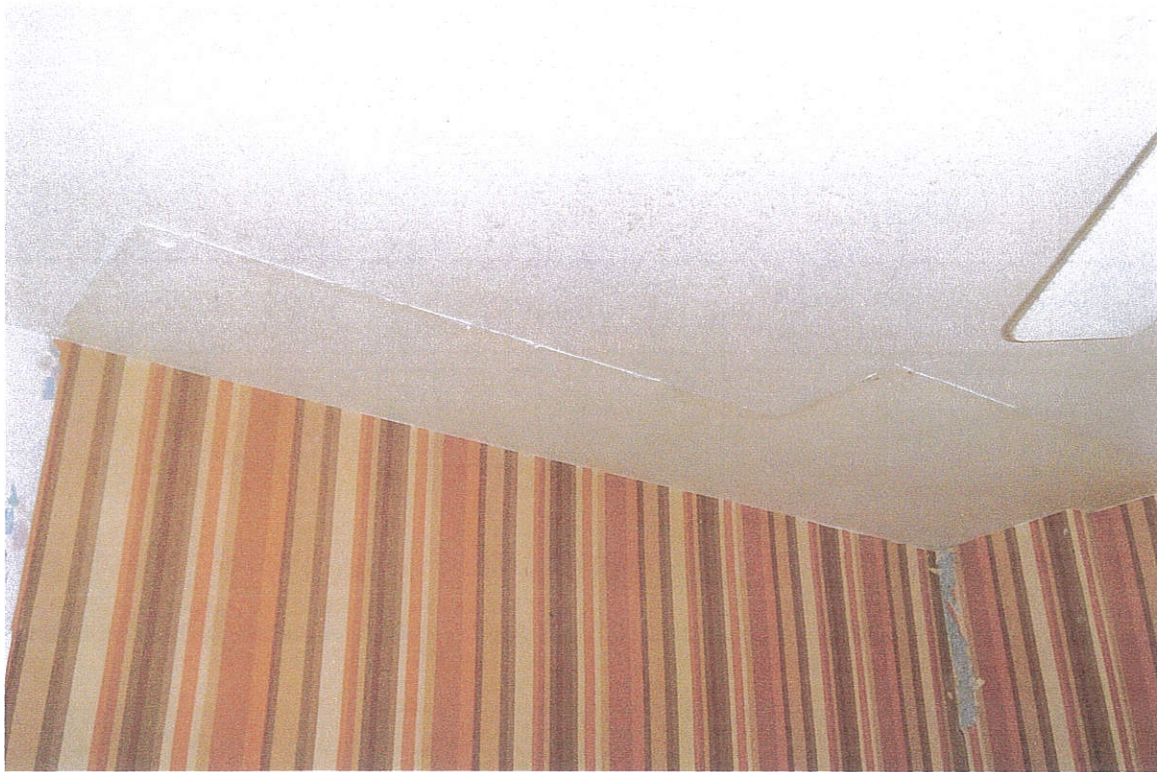
Kitchen Ceilings after trespasser Removed and stole kitchen cabinets
