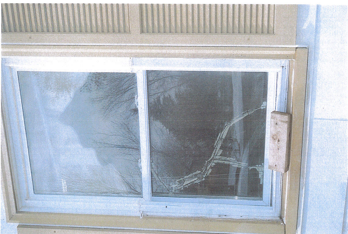
East living room window - Glass broken by trespasser. When he removed and stole window air conditioner
