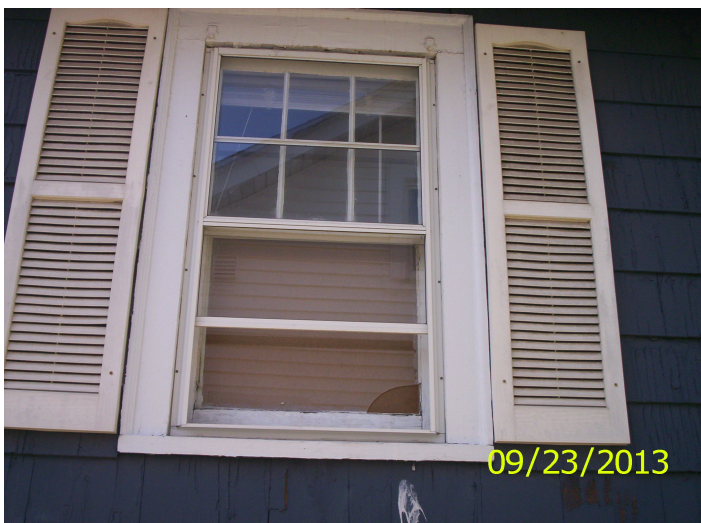
Boarded east side window
