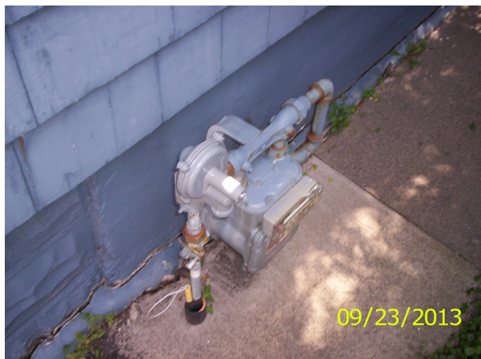
Gas meter locked off
