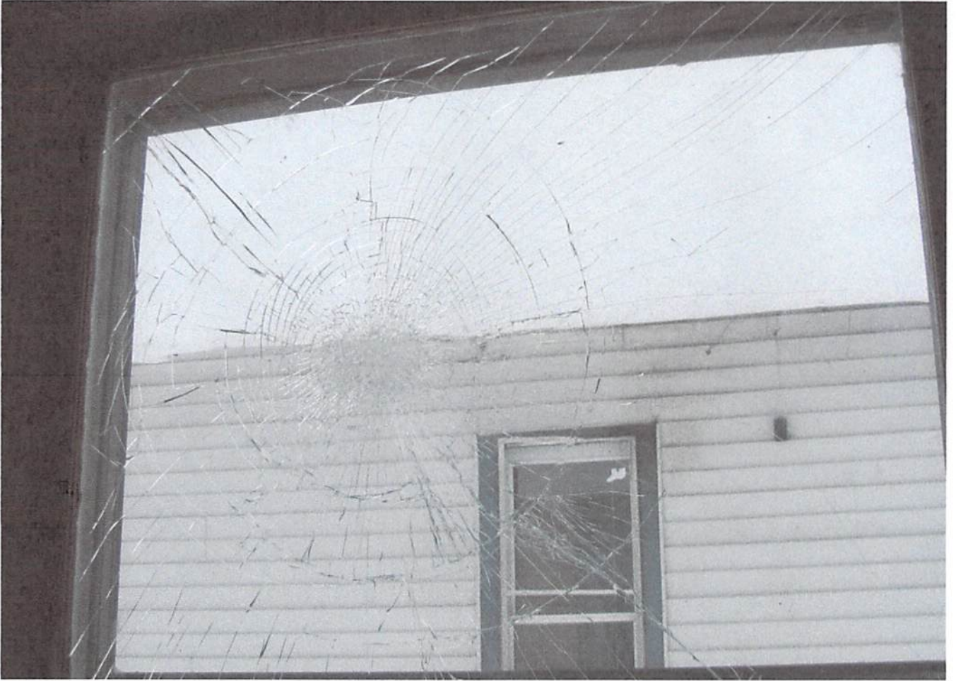
1st floor broken window
