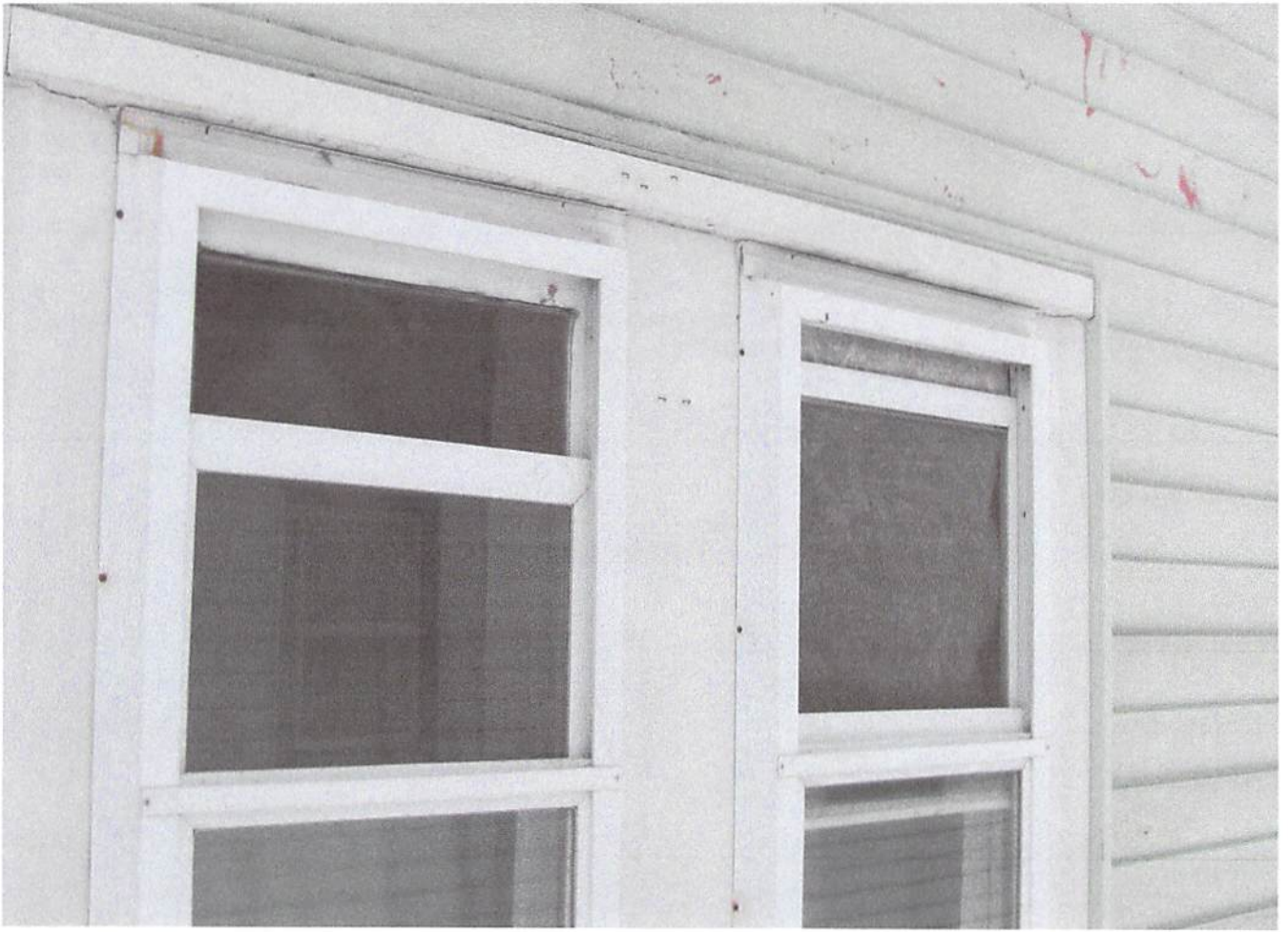
1st floor Broken windows
