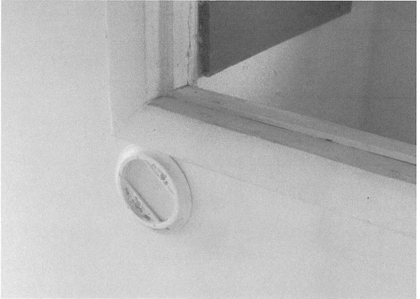
Smoke detector removed
