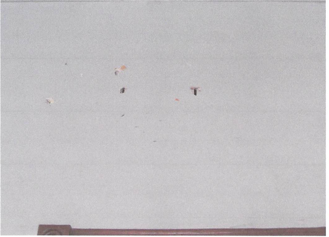
1st floor broken walls
