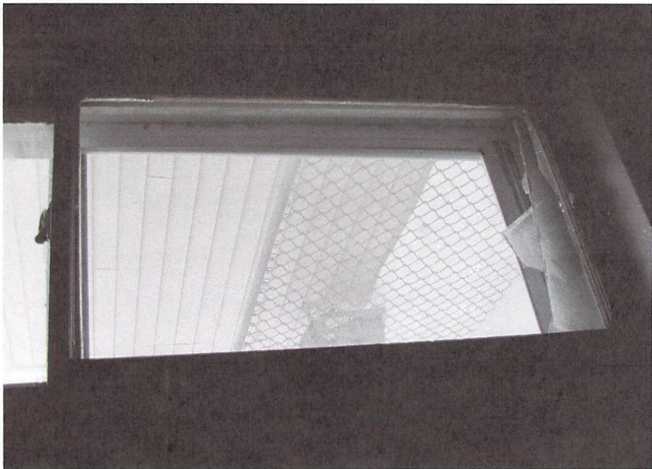
1st floor broken windows
