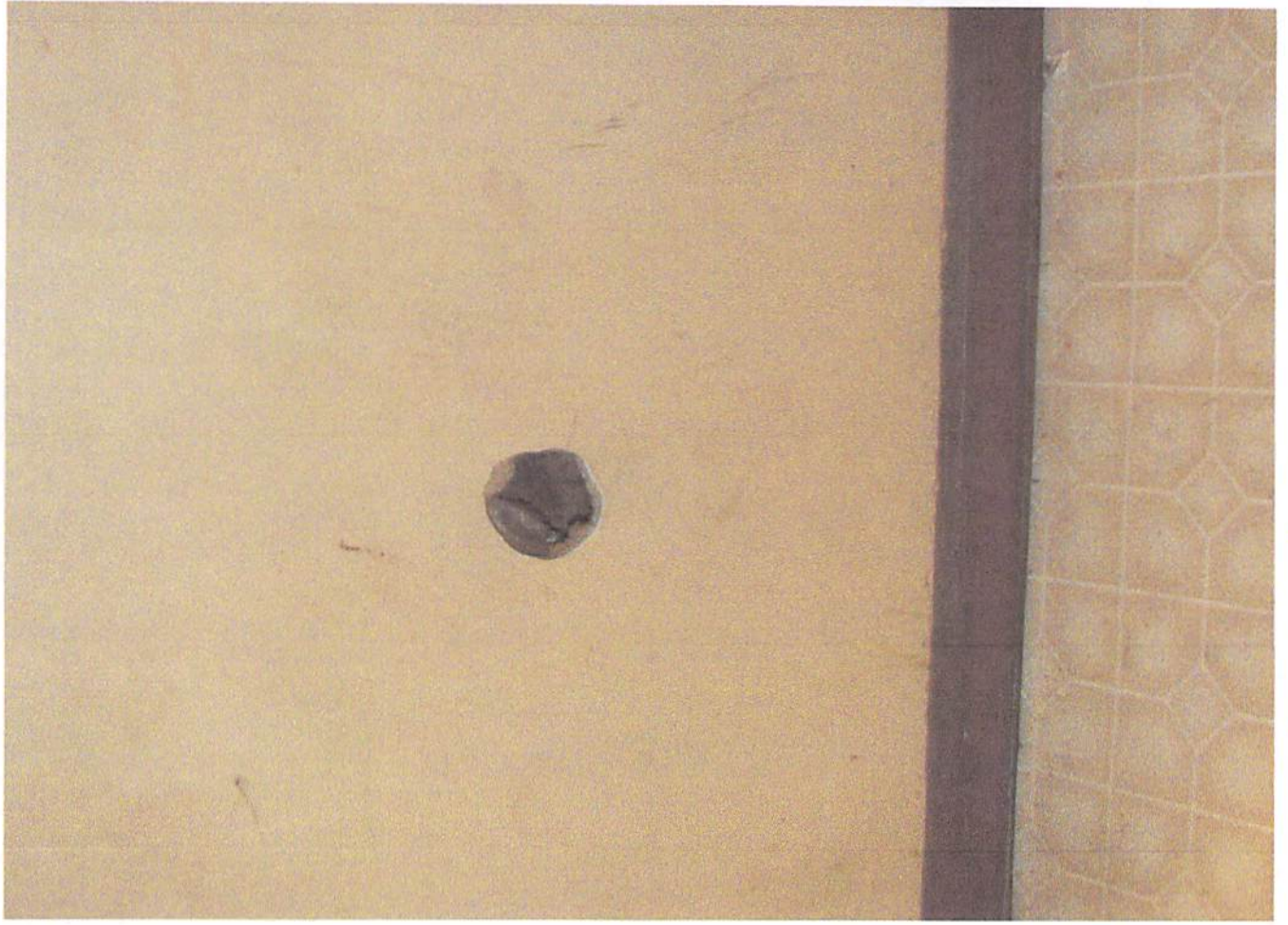
1st floor busted walls
