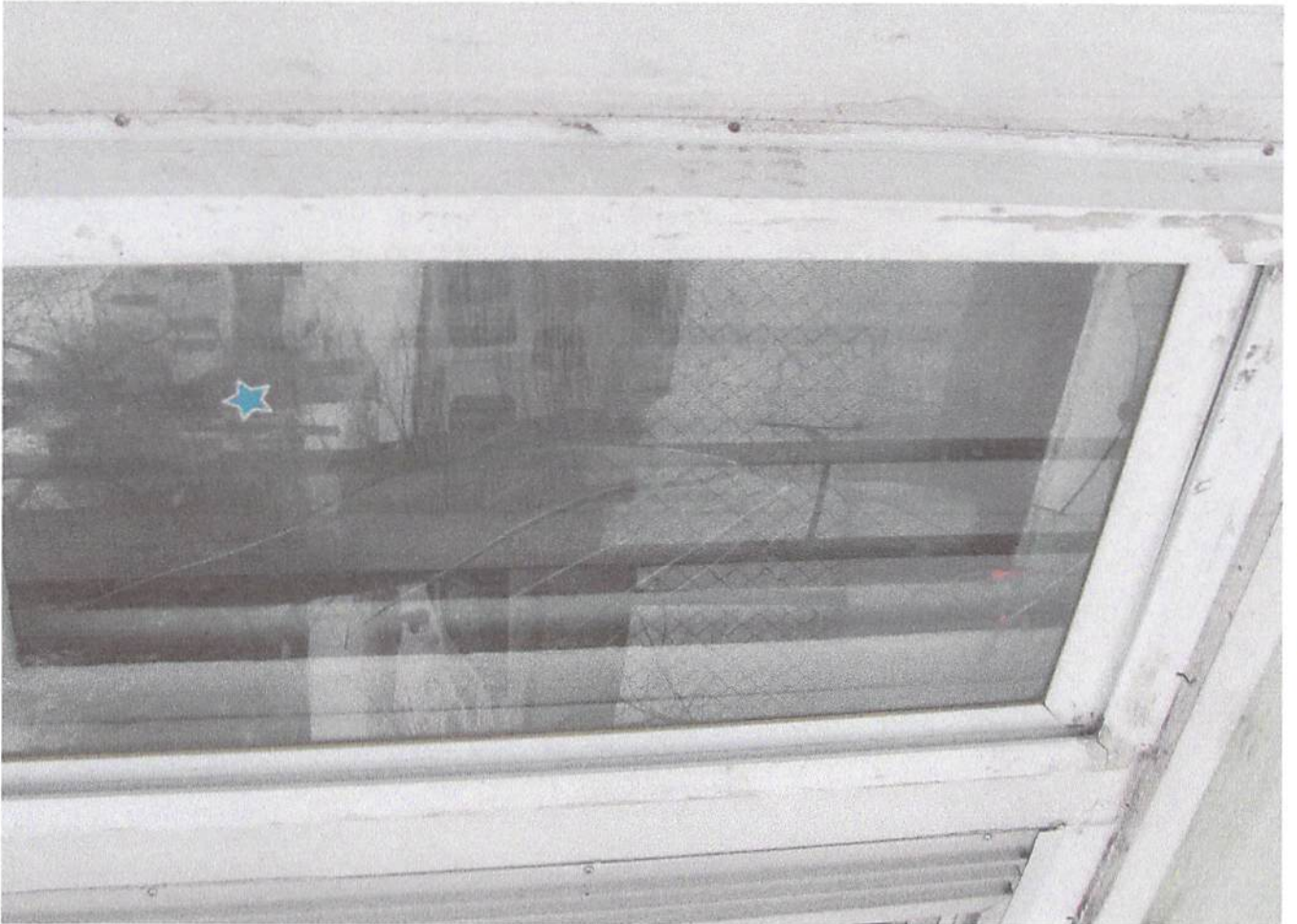
First floor Broken
