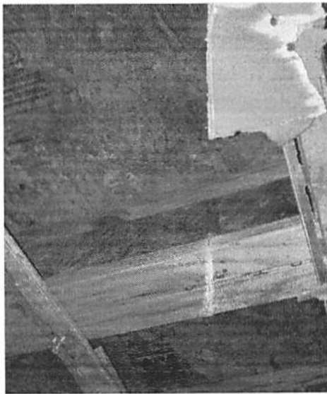
Figure 2: Damaged Wood I-Joists - To be Replaced
