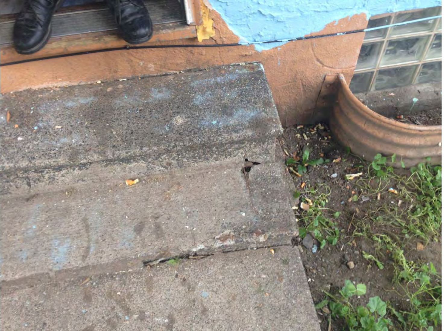
Deteriorated front steps, exposed rebar
