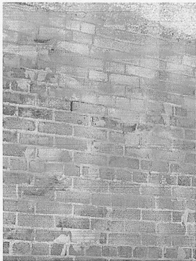
Photograph 2: "Classic" Freeze/Thaw Damage —Low to the ground, not very exposed to rainwater and in really bad shape. It turns out that this is a "bad" brick with a low S_{mf} .
