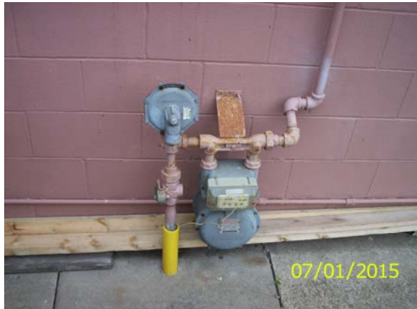
Gas meter locked off
