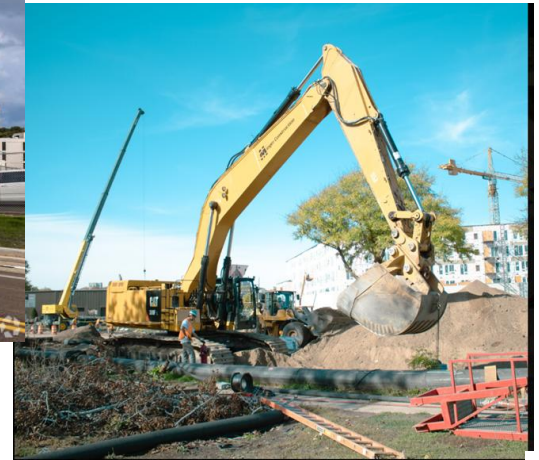
Water Street Sanitary Sewer Lift Station
