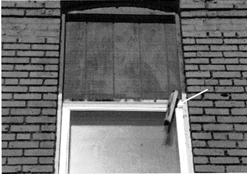
Six (6) upper units of windows must be patch or repaired
