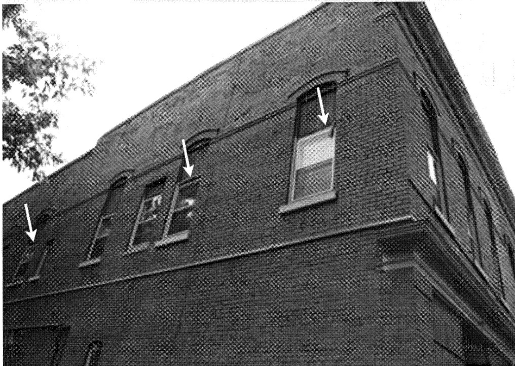
This depicts three (3) of the (6) upper window trim brick moulding which we are to be repaired or trim replaced.
