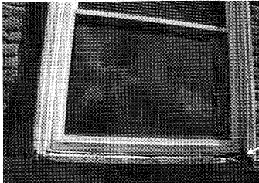
Nine (9) of the window sills must be patched or repaired. The one here needs to be replaced.
