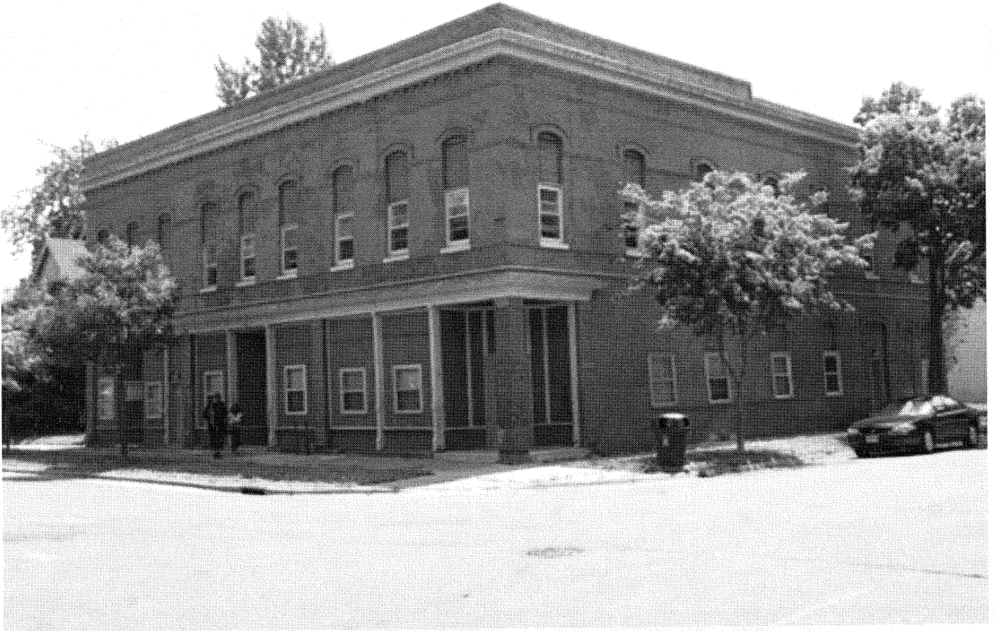
Lafond Apartments at 434 LaFond Avenue Masonry repairs are to be made at specific areas
