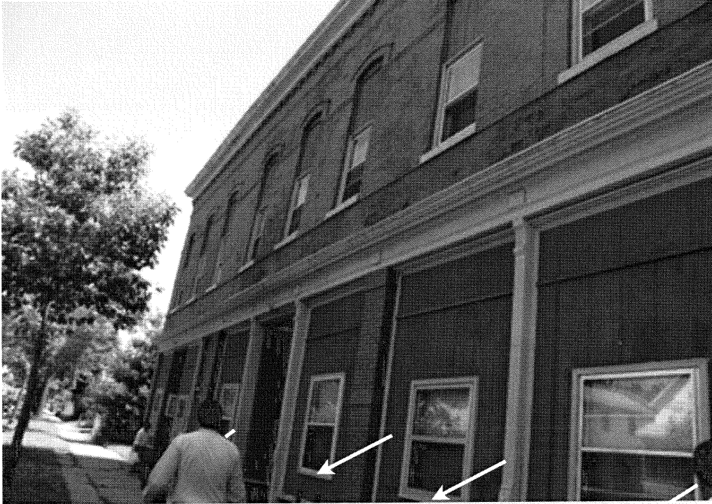
Four (4) of the nine (9) window sills that will be repaired or replaced are shown here.
