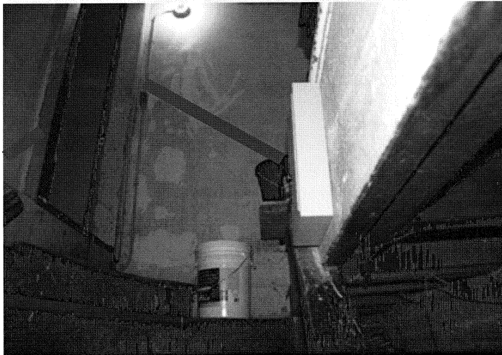
One handrail to be installed at the top of stairs, 36 inches above stairway
