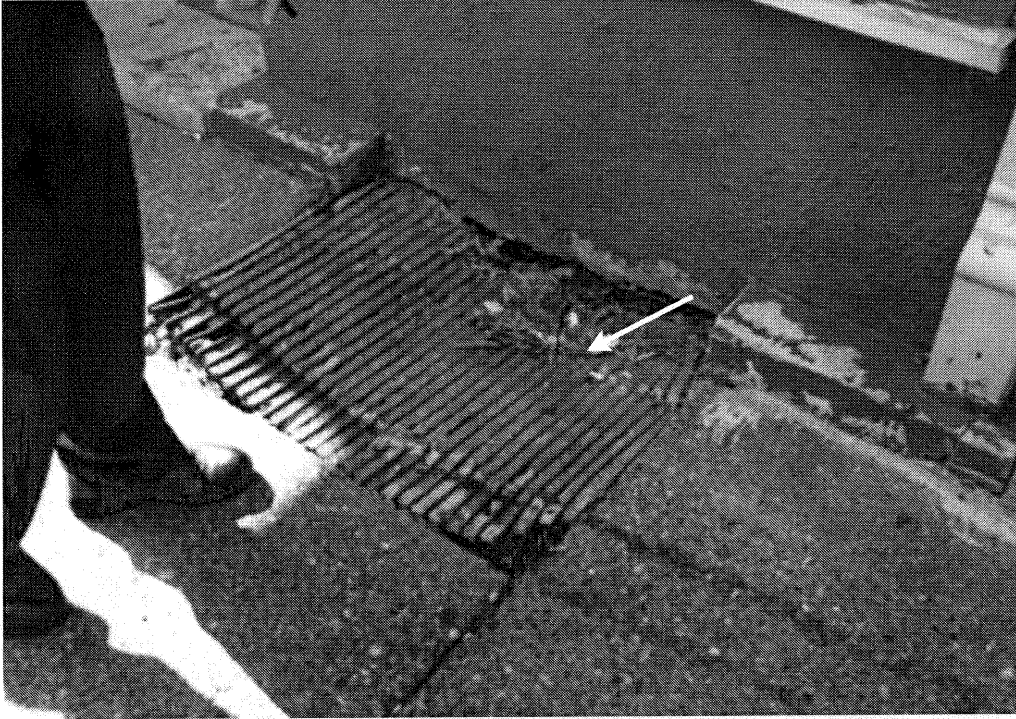
This grate will be removed and the sidewalk will be poured in its place to provide a smooth surface.
