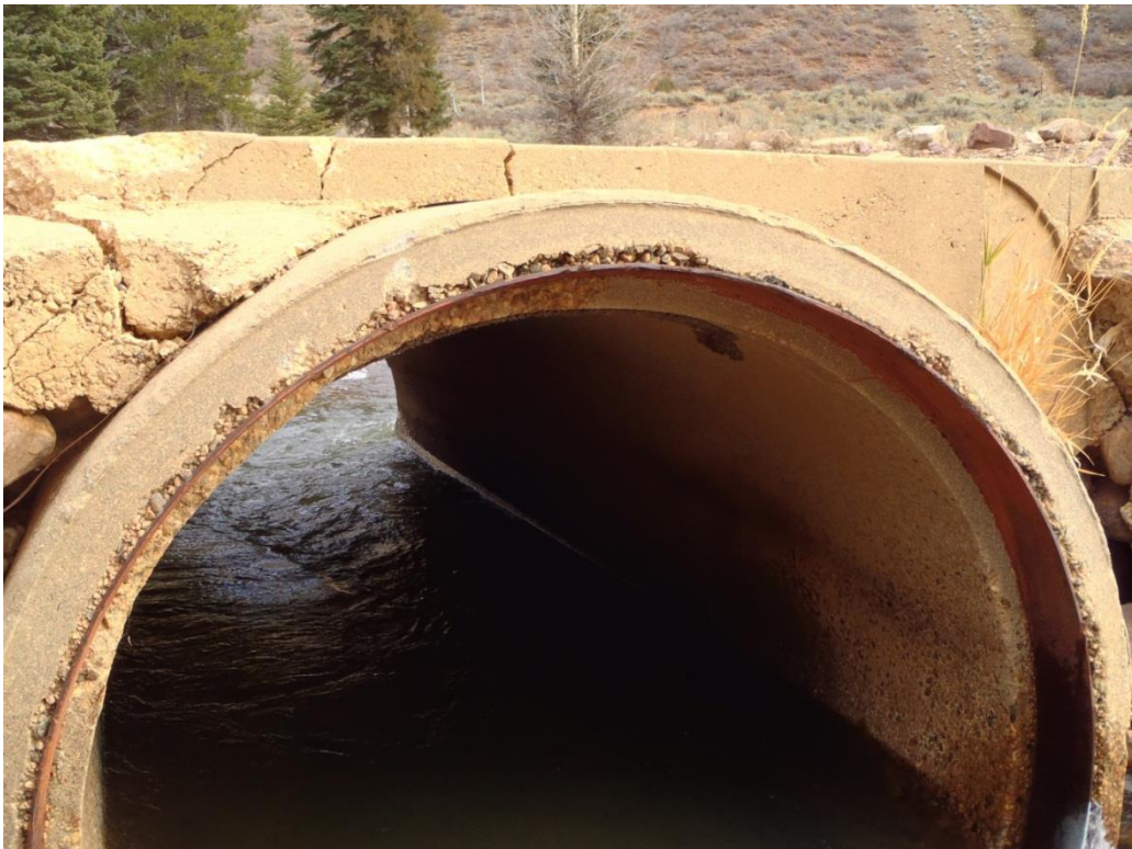
Figure 4 –Honeycombed Mortar Around Joint Ring of Surplus PCCP.
