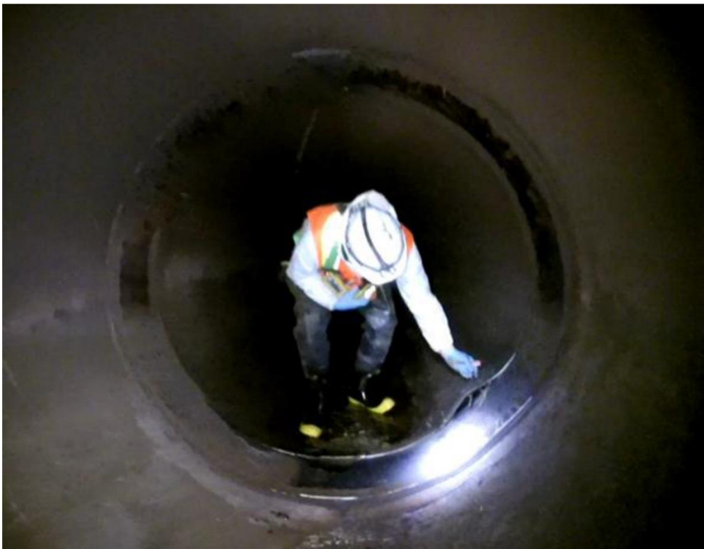
Figure 9: Joint MH.28A-J29: WEKO Seal with “Sprung” Retaining Band.
