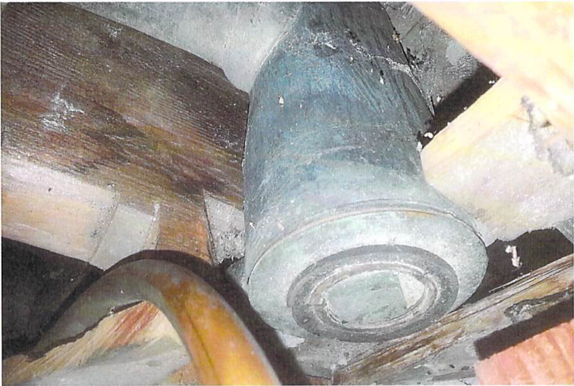
UPSTAIRS Bathroom plumbing
