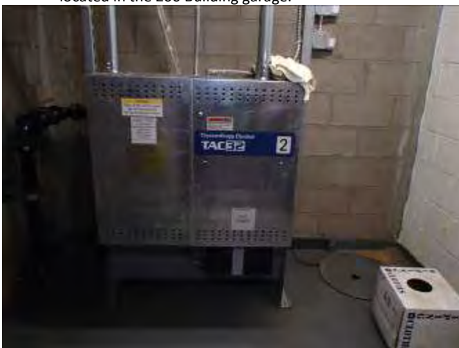
17. Elevator motor for the elevator within the 215 Building, located in the 215 Building garage.
