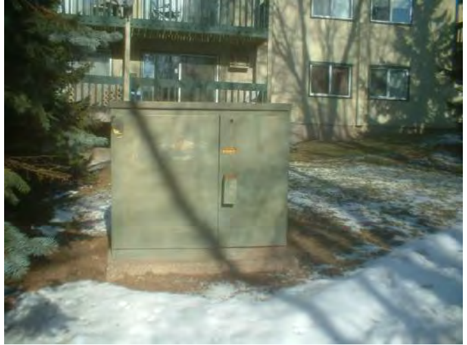
Photo 2 – Typical pad-mounted transformer
