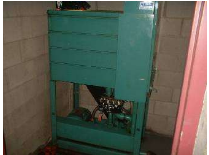
Typical elevator machinery
