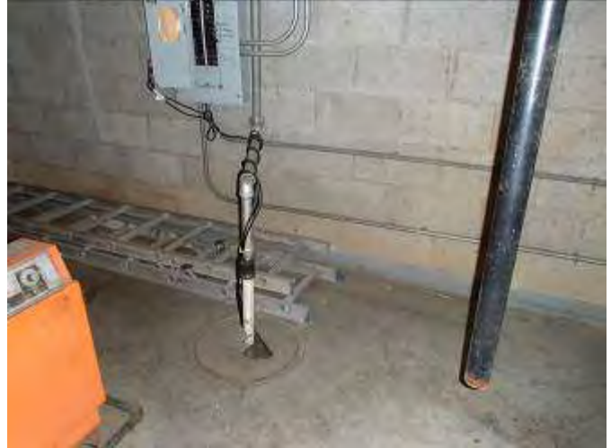
14. Sump in the boiler room.
