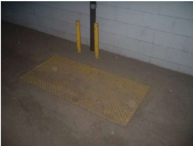
Photo 3 – Oil/water separator cleanout port in garage area
