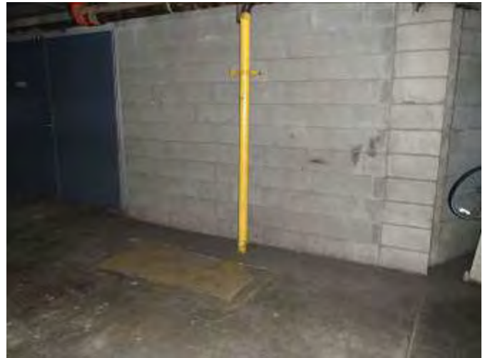
16. Oil/water separator cleanout in the 215 Building garage.
