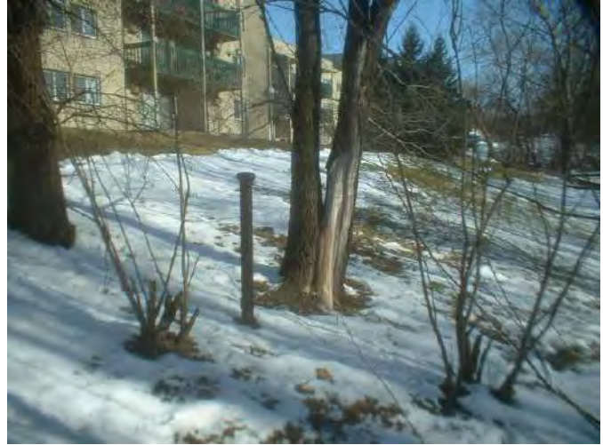
Photo 8 – Vent pipe south of building for 30,000 gallon heating oil UST
