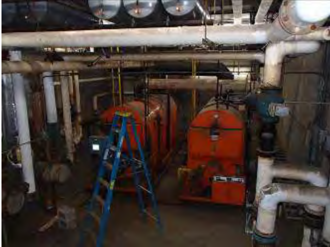
13. Boiler room located in the 200 garage.
