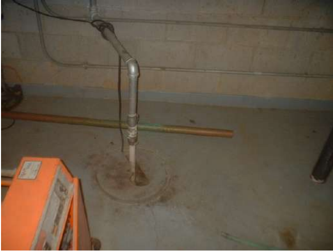
Photo 7 – Typical sump pump installation
