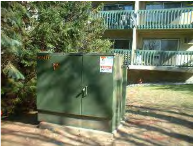
Typical pad-mounted transformer
