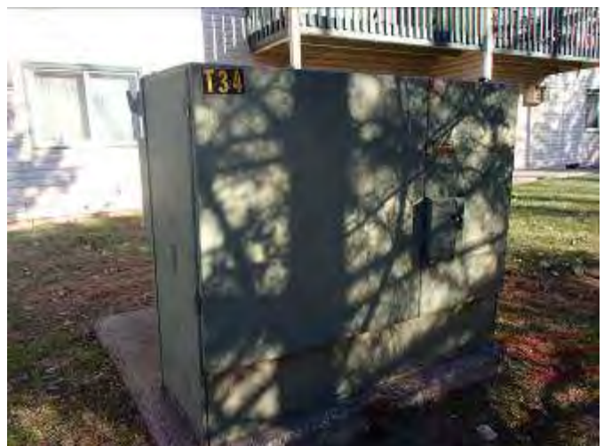
24. One of six pad-mounted transformers located around the building.
