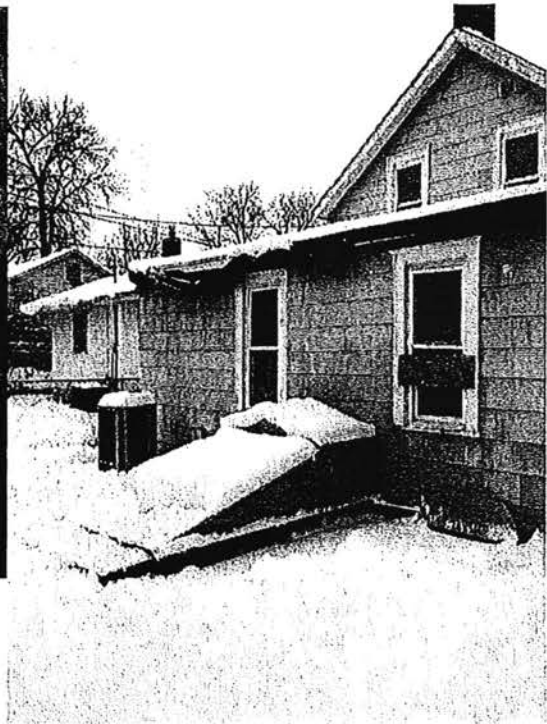
Photo 6 – Uninsulated, Unprotected Exterior Stair Access
