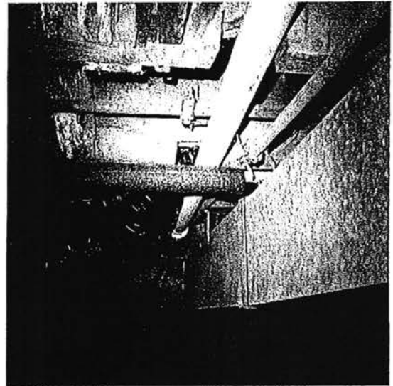
Photo 10 – Notched Floor Joists
