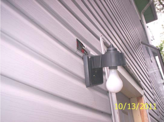
Unfinished south side light fixture
