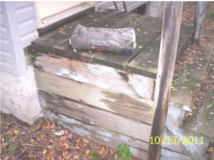
Rot damaged rear steps
