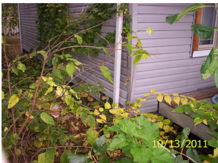
North side unfinished and unapproved siding installation
