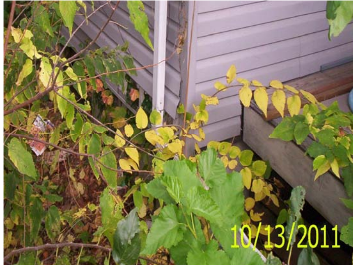
North side unfinished and unapproved siding installation
