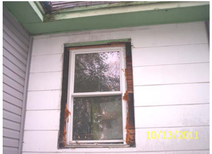
East side unfinished window installation
