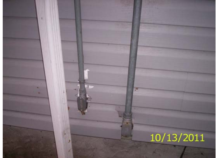
South side unapproved siding installation
