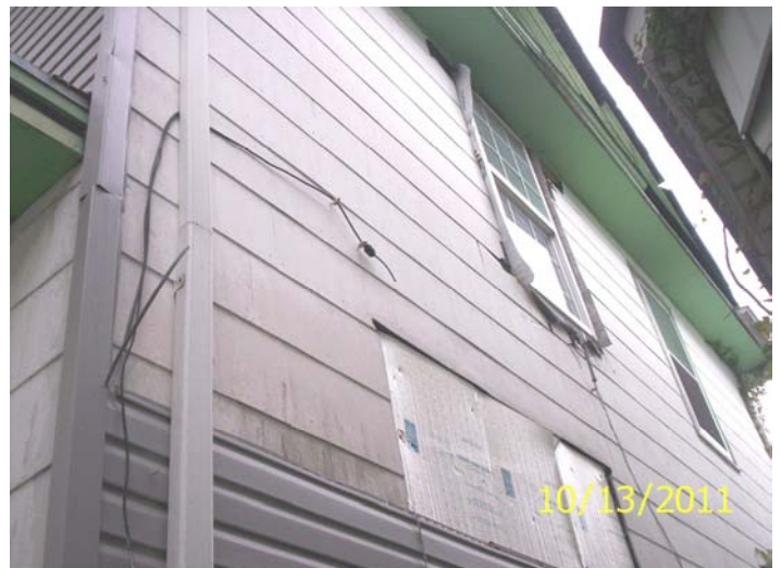
North side missing siding, abandoned window
