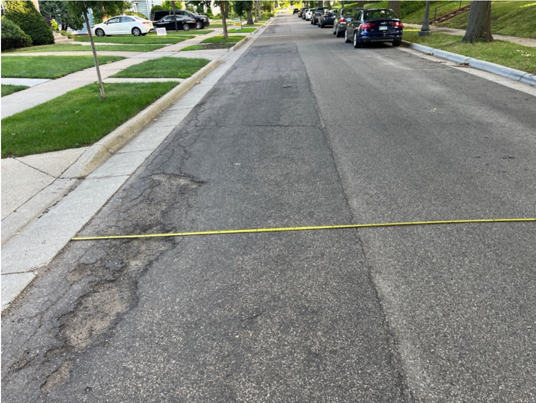
1) View looking south at unreconstructed east lane of pavement (the driving lane), which is full of potholes. Full-width reconstruction is visible at each manhole.
