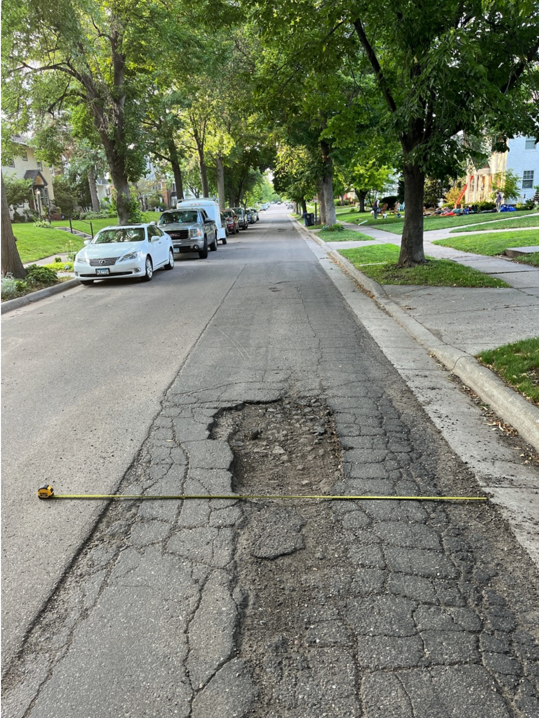
3) View looking north at unreconstructed east lane of pavement (the driving lane due to parking restrictions), which is full of potholes. Full-width reconstruction is visible at each manhole.
