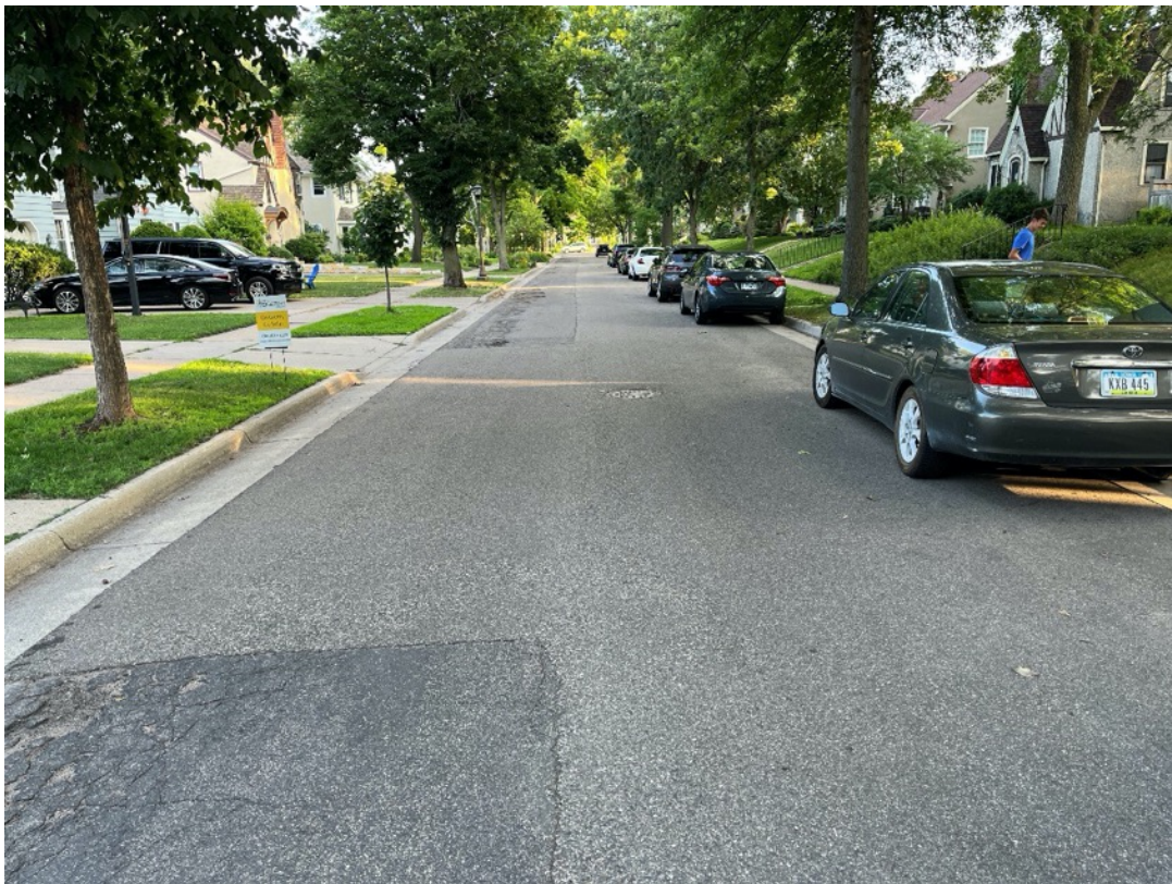
2) View looking south at fully reconstructed pavement around manhole in excellent condition, preceded and followed by unreconstructed pavement in poor condition.
