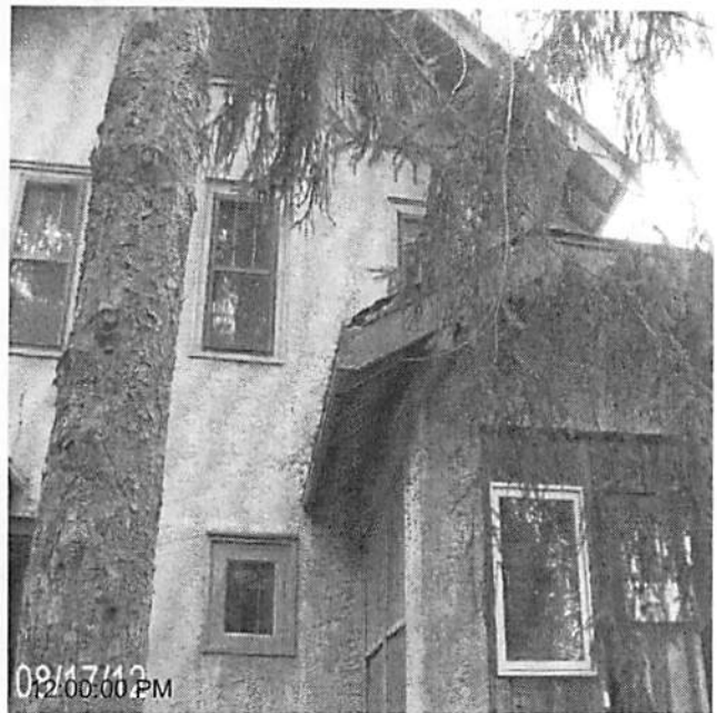
Date Completed: before: repair rotted fascia front entrance
