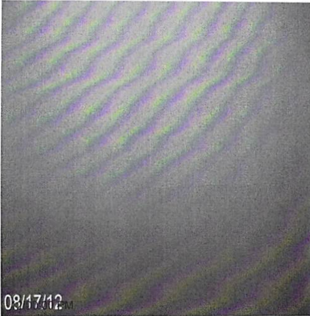
Date Completed: before: repair cracks in ceiling
