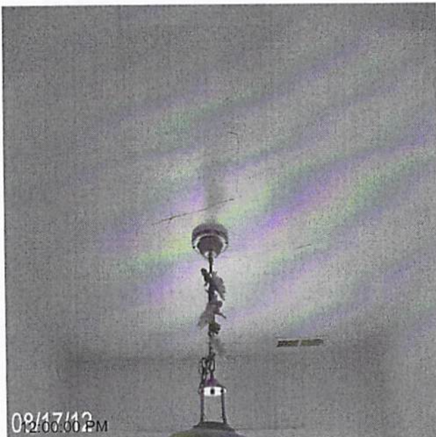
Date Completed: before: repair cracks in ceiling
