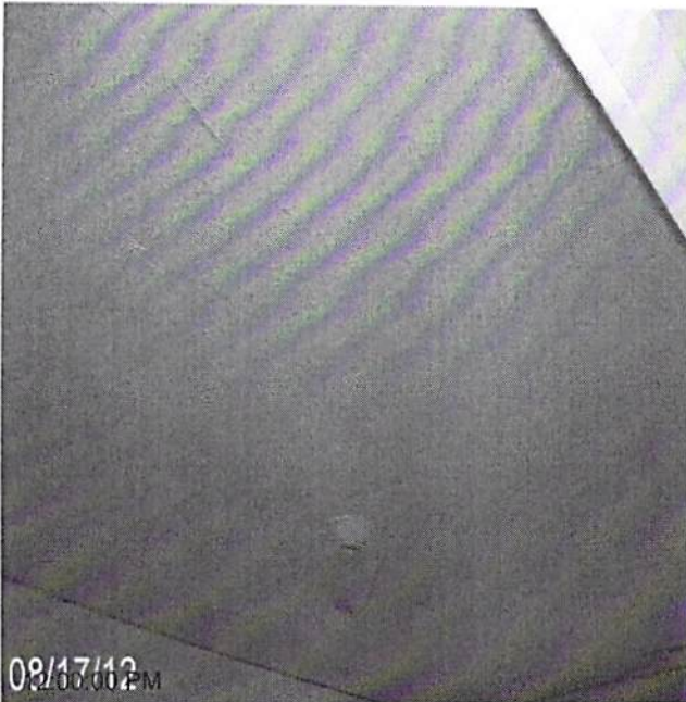
Date Completed: before: repair cracks in ceiling
