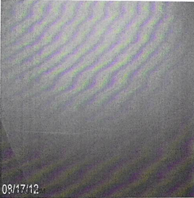
Date Completed: before: repair cracks in ceiling
