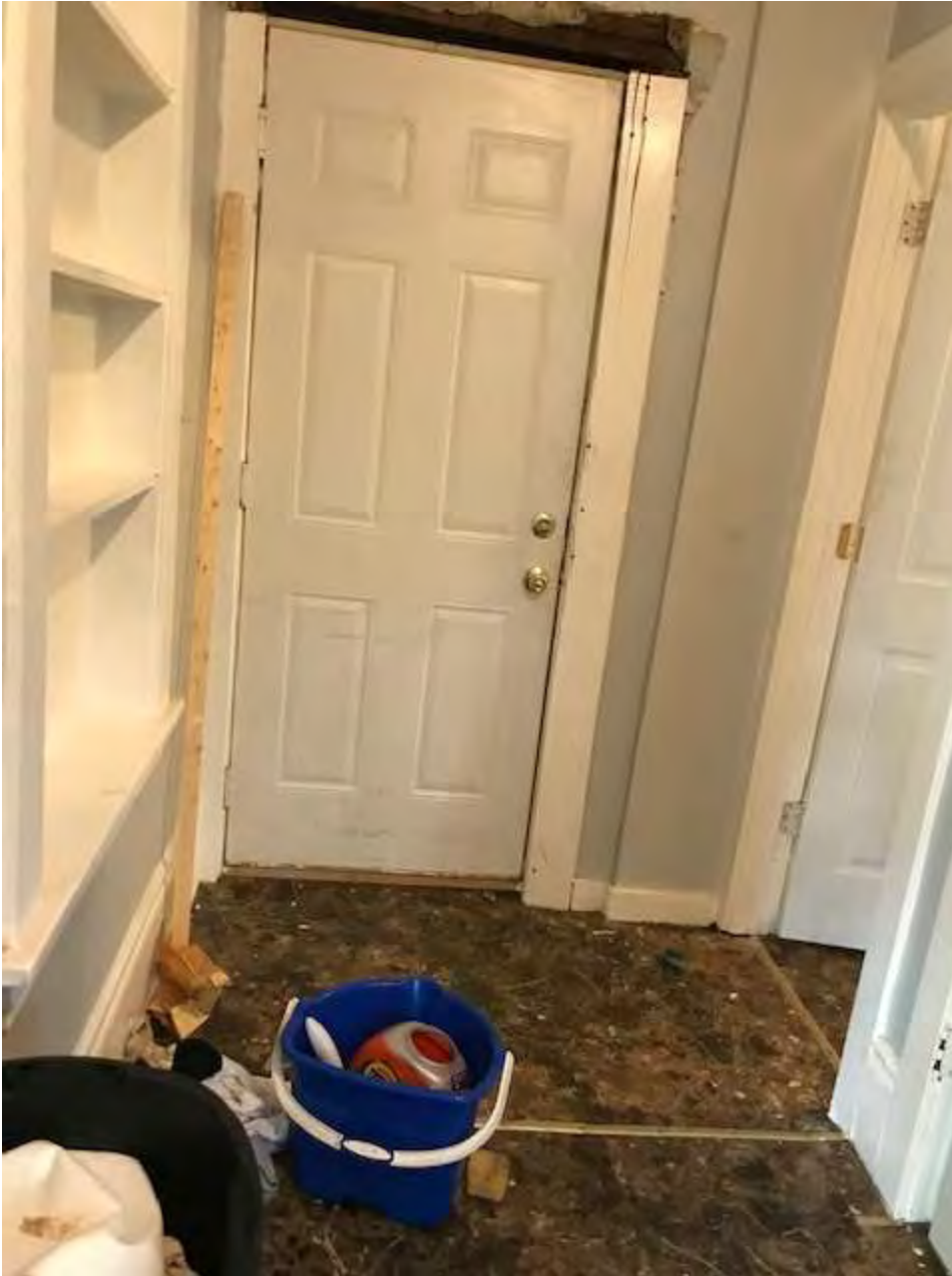
The door leads to the upper level Unit (2) – was unopenable during initial inspection.
