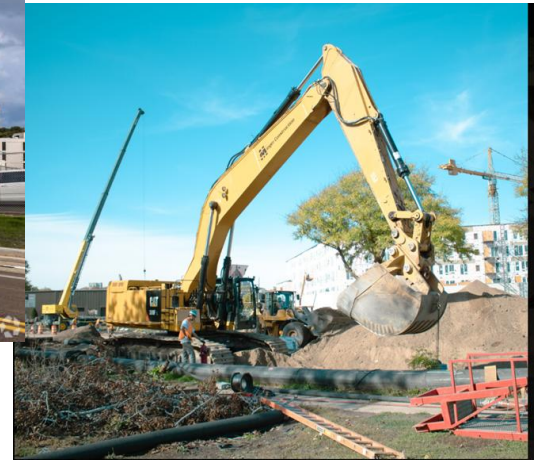
Water Street Sanitary Sewer Lift Station
