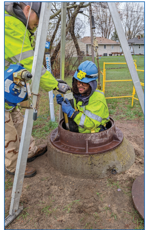
Christopher Robinson pulls himself up from out of a 60-inch conduit while Erik Sorenson supports the ladder. The two were on hand to assist the office of technology and communications film Eric Noe in the conduits while talking about being an engineer for SPRWS for an upcoming jobs video on the position. The filming took place on Monday, April 29.
