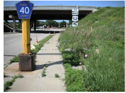
View west of sidewalk and signal at TH 52 bridge and E. Lafayette frontage road.
