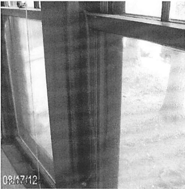
Date Completed: before: replace broken sash cords 1st floor living
