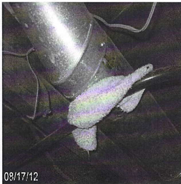
Date Completed: before: replace heating register
