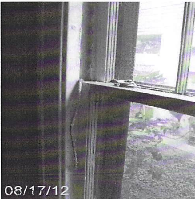
Date Completed: before: replace broken sash cord upstairs bedroom
