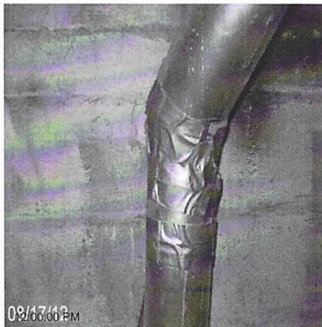
Date Completed: before: replace heating register
