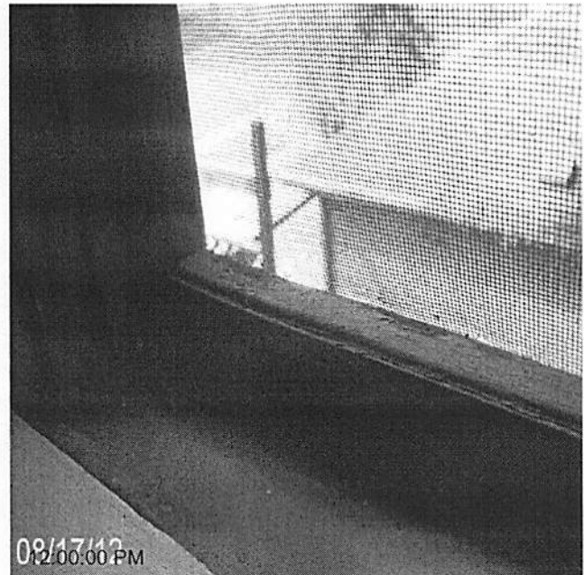
Date Completed: before: replace storm window
