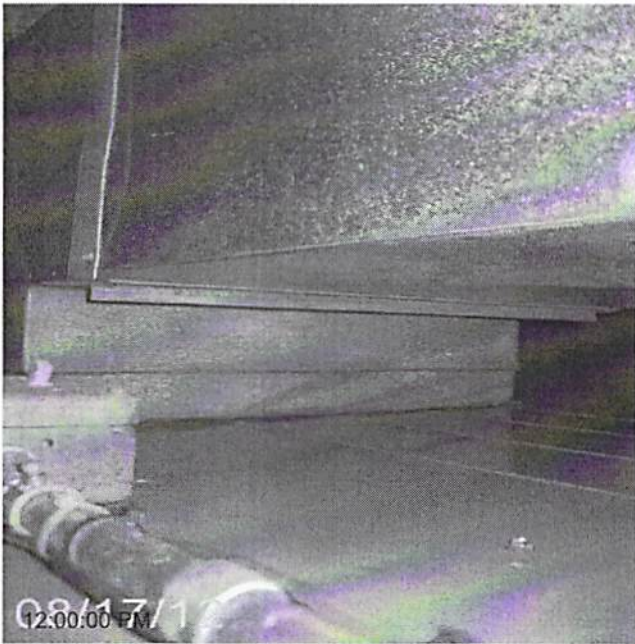
Date Completed: before: replace heating register
