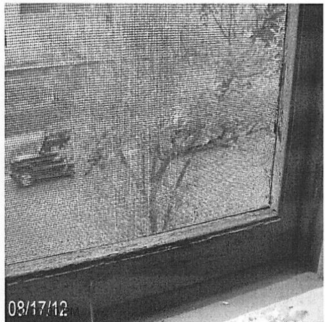
Date Completed: before: replace storm window
