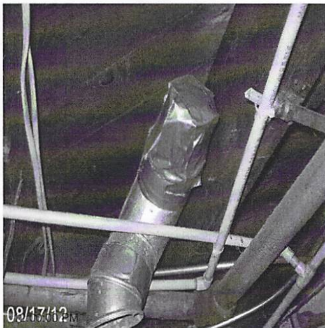
Date Completed: before: replace heating register
