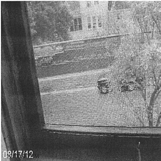
Date Completed: before: replace storm window
