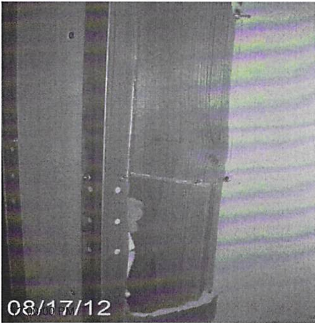
Date Completed: before: repair unfinished sheetrock
