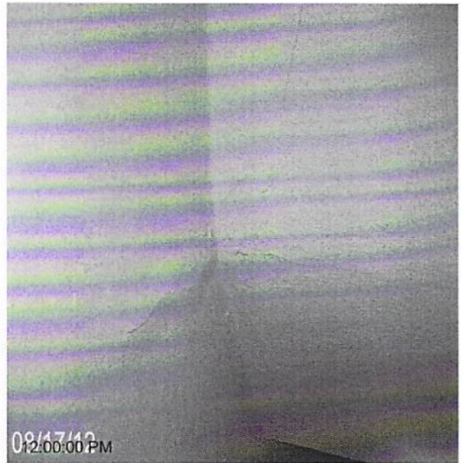
Date Completed: before: repair unfinished sheetrock
