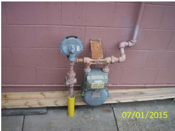
Gas meter locked off
