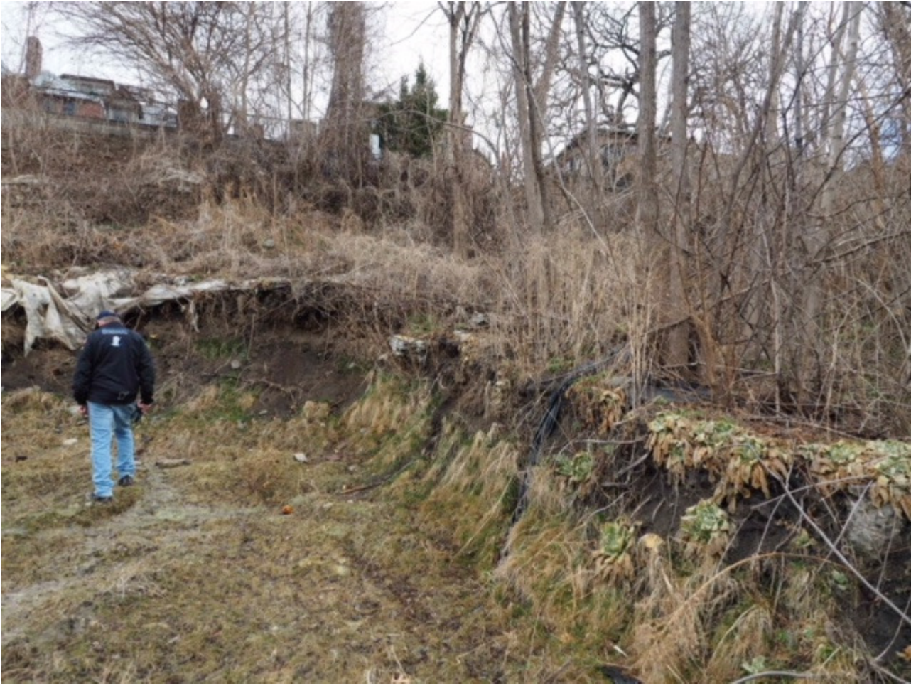
Vertical cut in slope below 322/324 Summit
