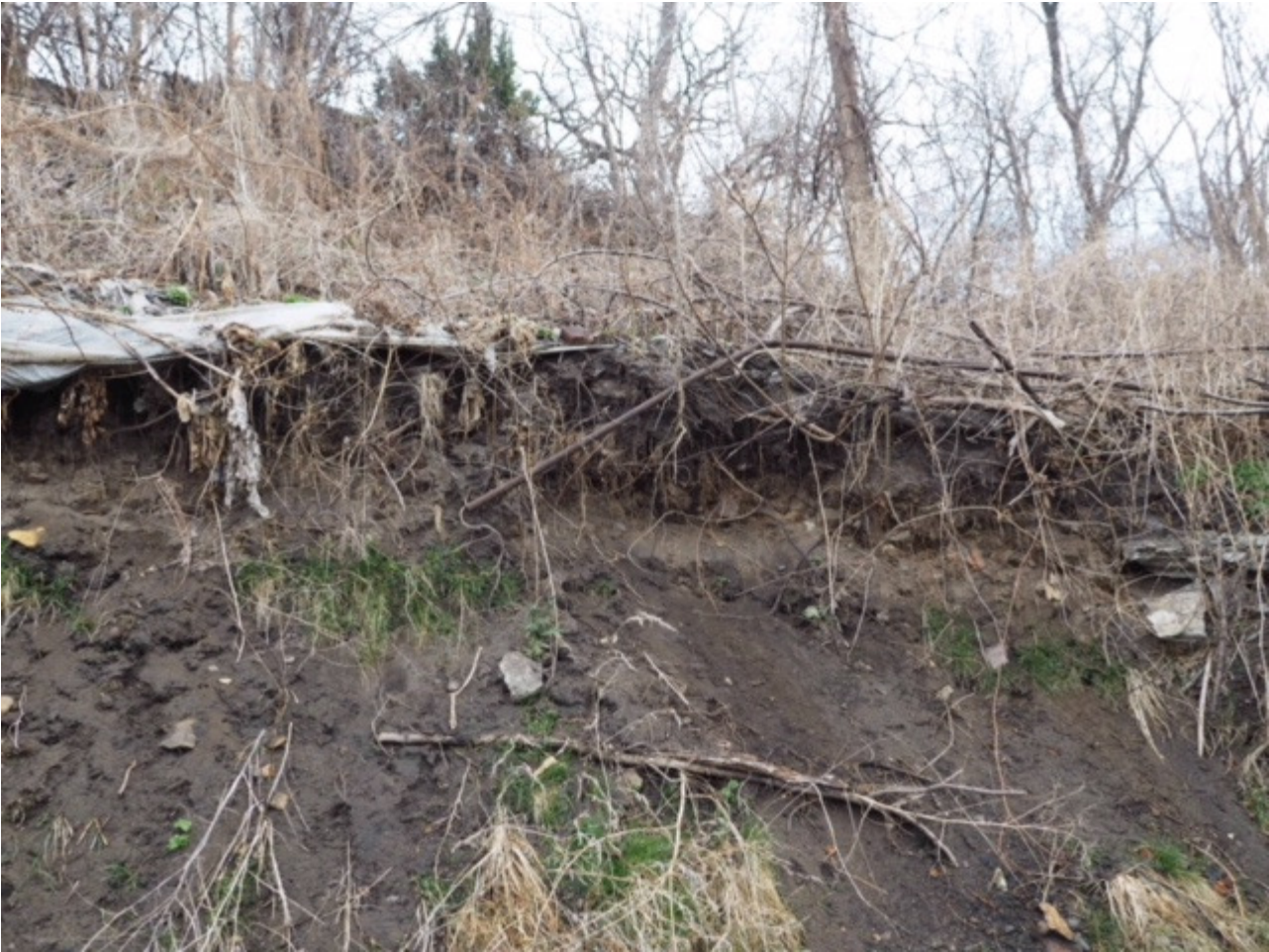
Unstabilized soil below 322/324 Summit
