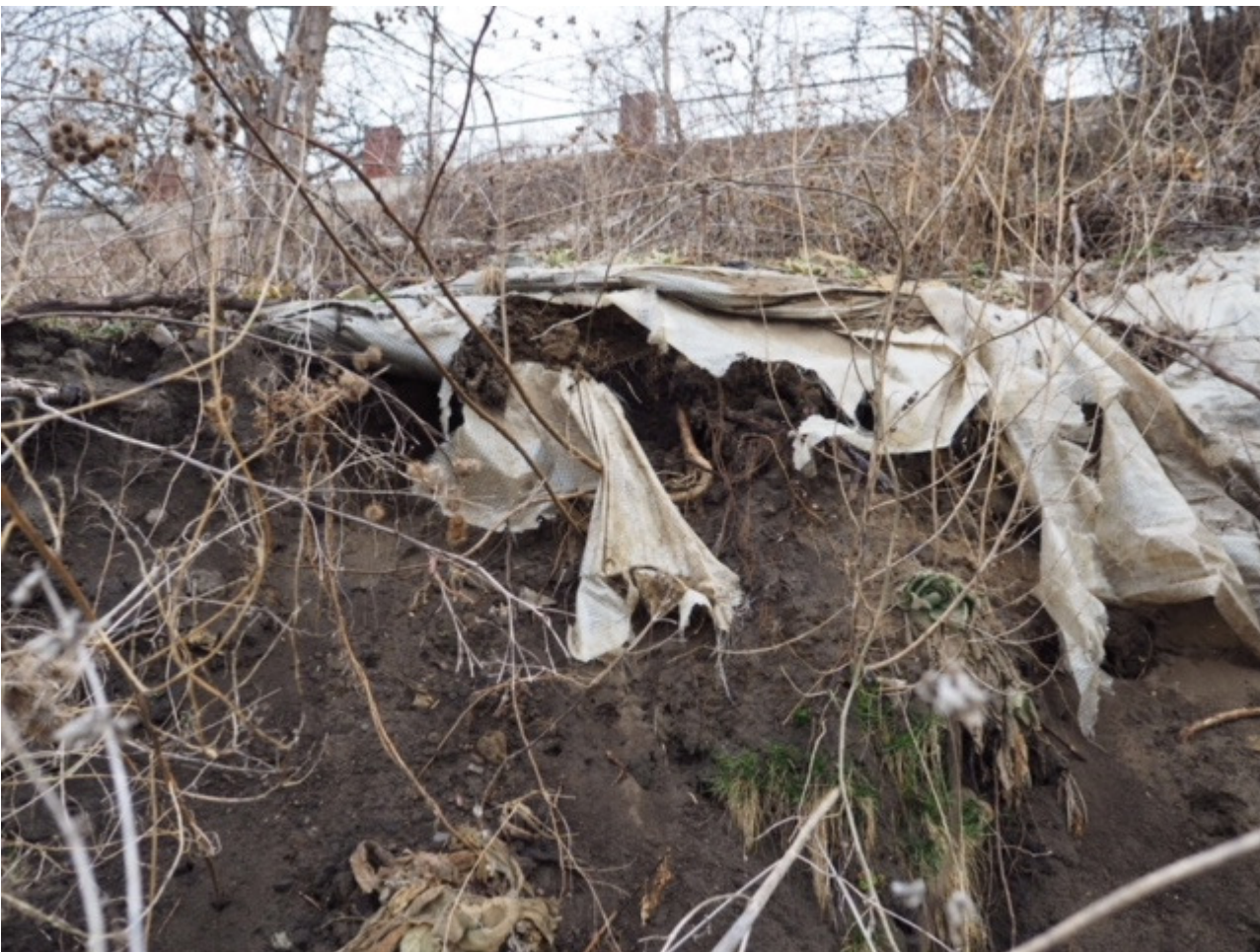
Backhoe destruction of soil retention fabric
