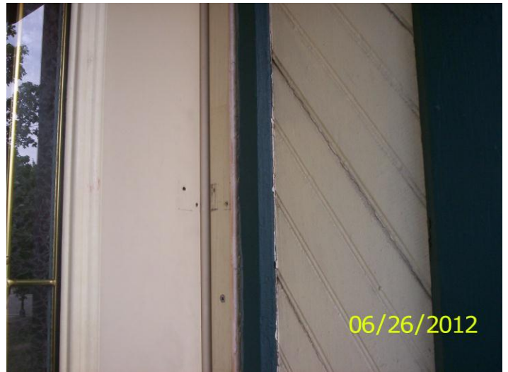
Upper markings from securing
