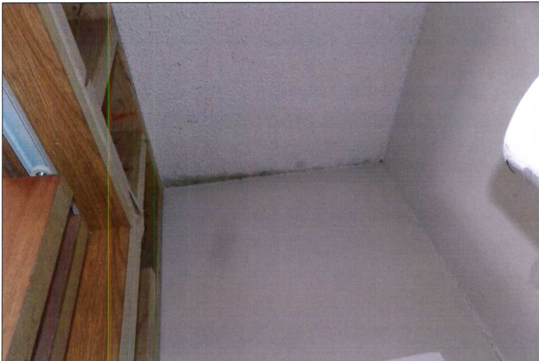
Photograph # 15: Water stains at wall/ceiling
