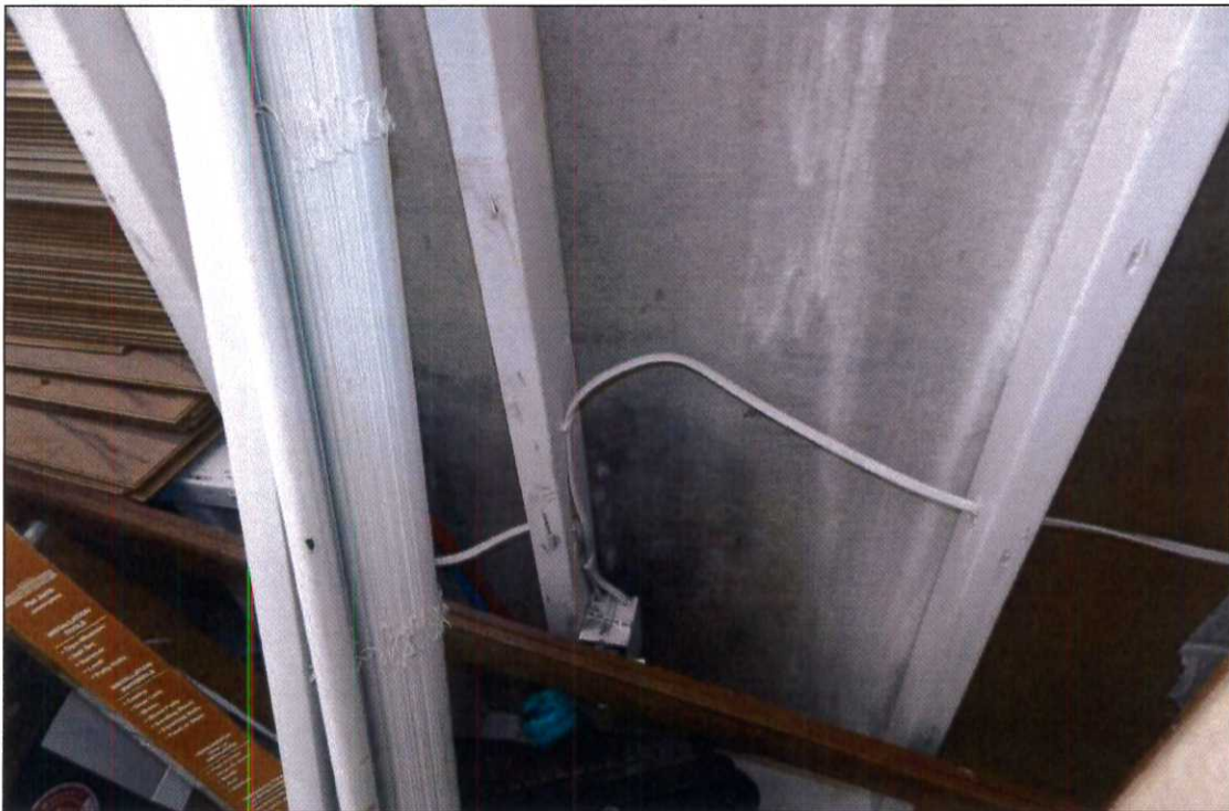
Photograph # 14 Bedroom – water staining on floor; Kilz applied to wall
