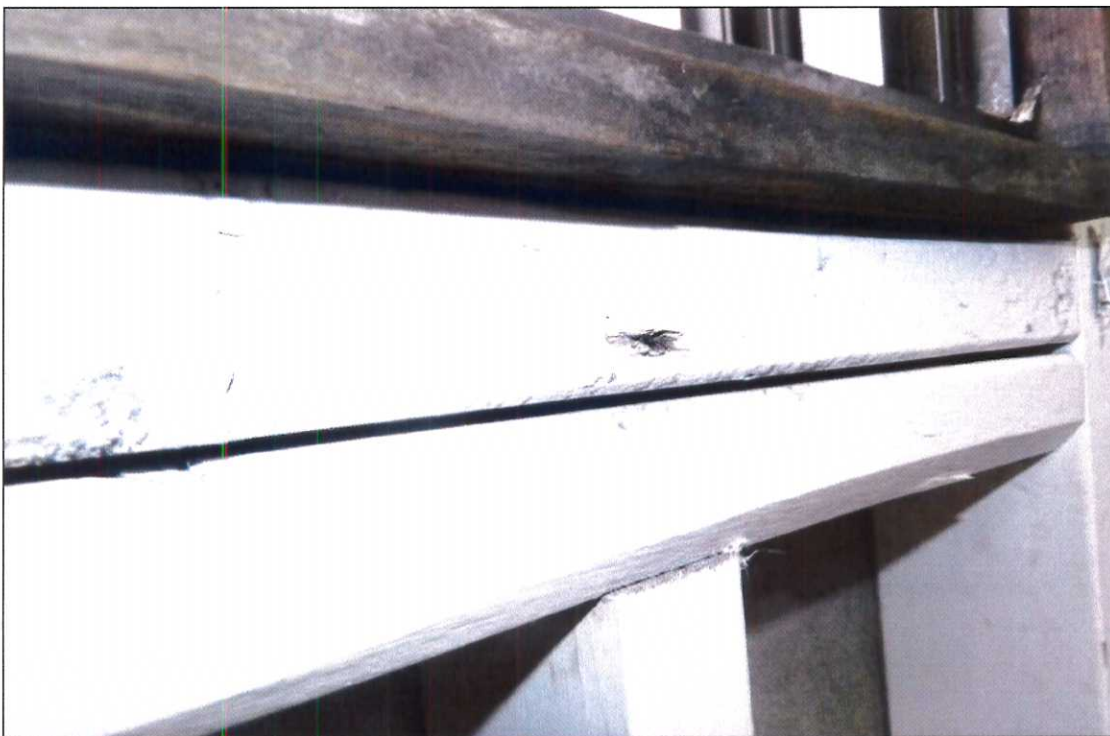
Photograph # 24: No flashing below window
