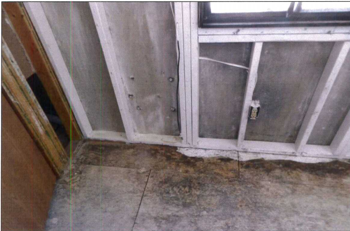
Photograph # 10: Bedroom – water staining on floor; Kilz applied to wall
