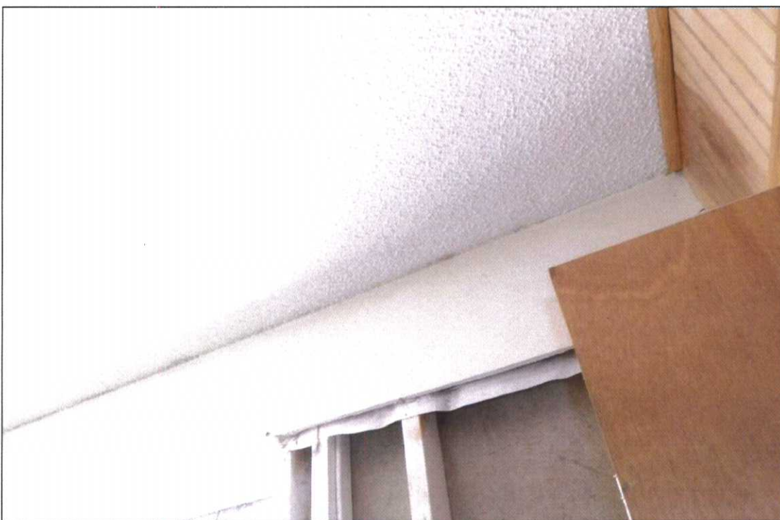
Photograph # 16: Water stains at wall/ceiling
