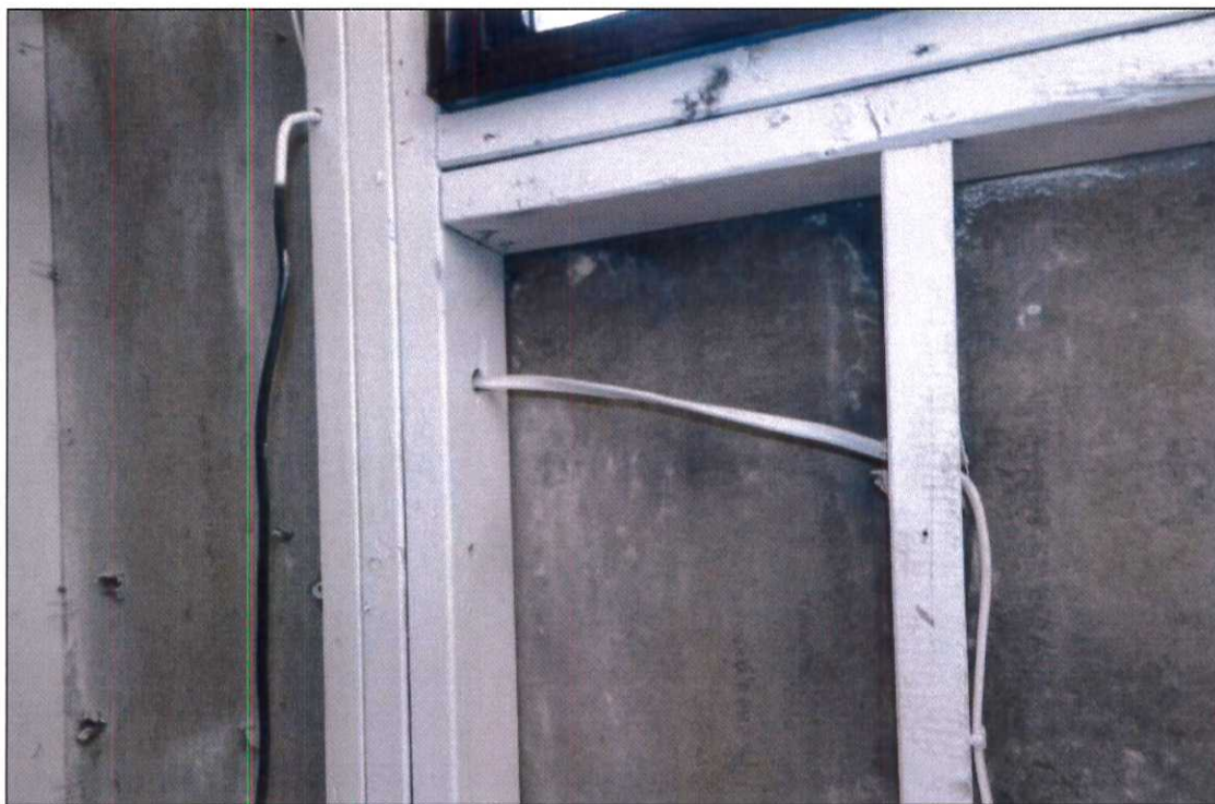
Photograph # 12: Bedroom – water staining on floor; Kilz applied to wall
