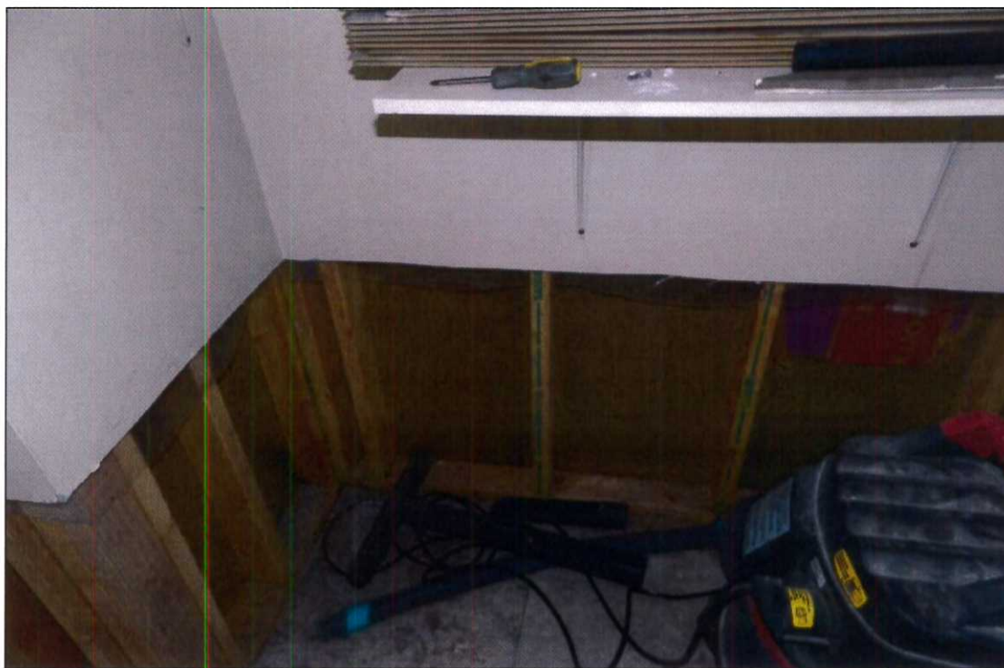
Photograph # 8: Water staining in bump-out across from bathroom
