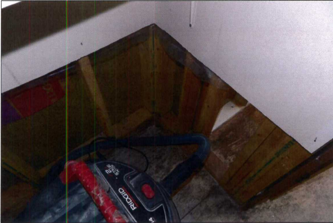
Photograph # 9: Water staining on floor in bump-out across from bathroom
