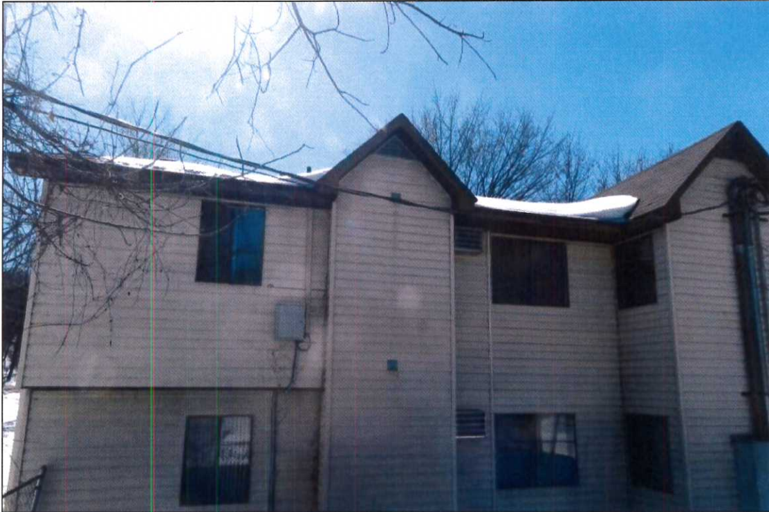
Photograph # 25: View of the 3 affected windows
