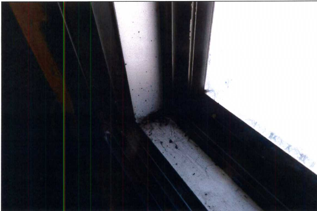
Photograph # 23: Deterioration at window jamb/sill intewrsection
