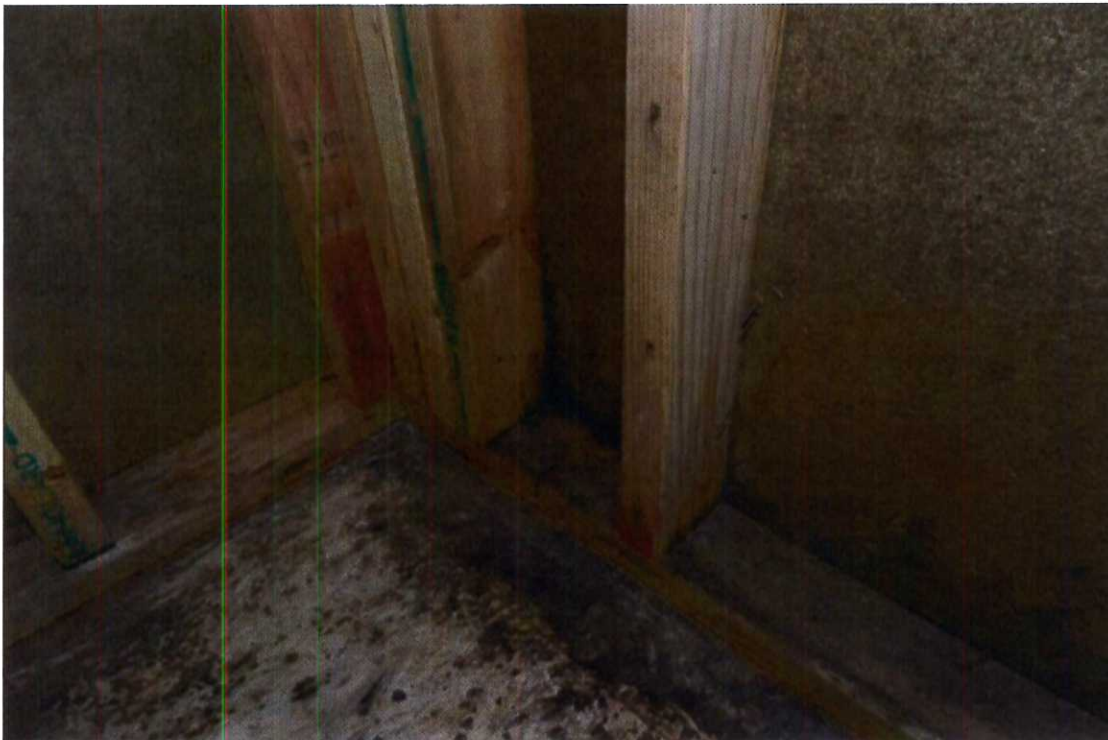
Photograph # 5: Close up of water staining below window in Photo 4
