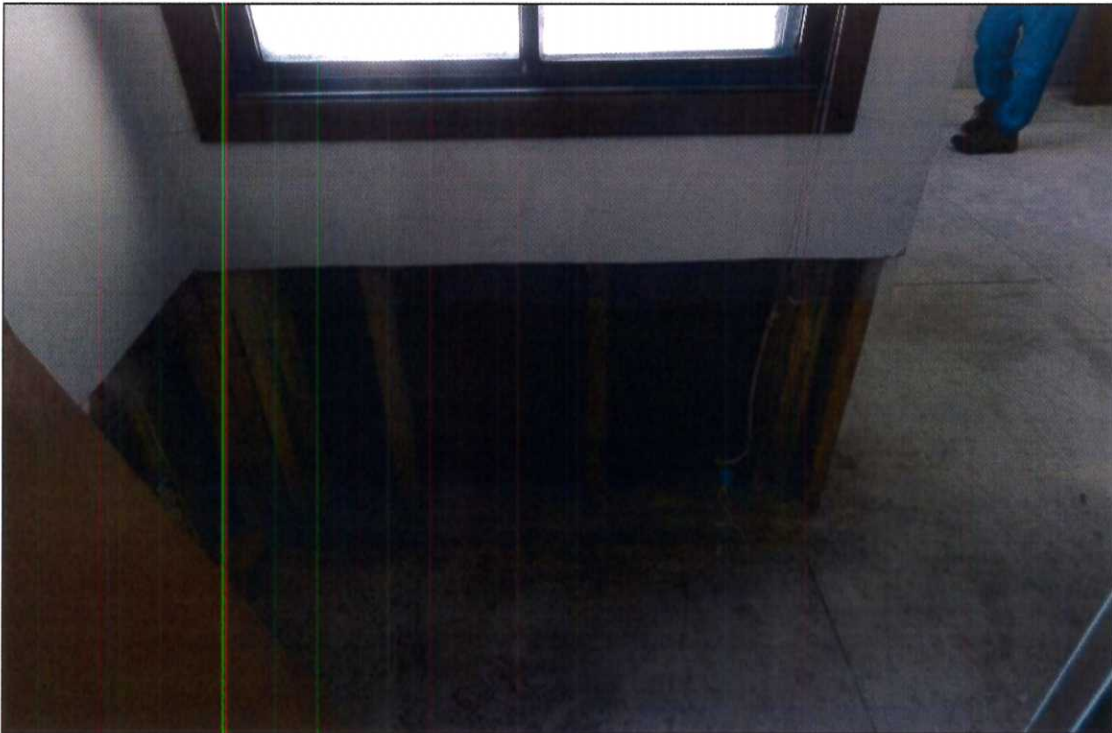
Photograph # 4: Water staining on floor below window to the west
