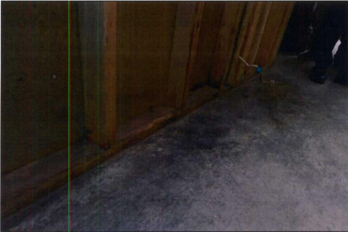
Photograph # 3: Staining on floor below the window in Photo 1
