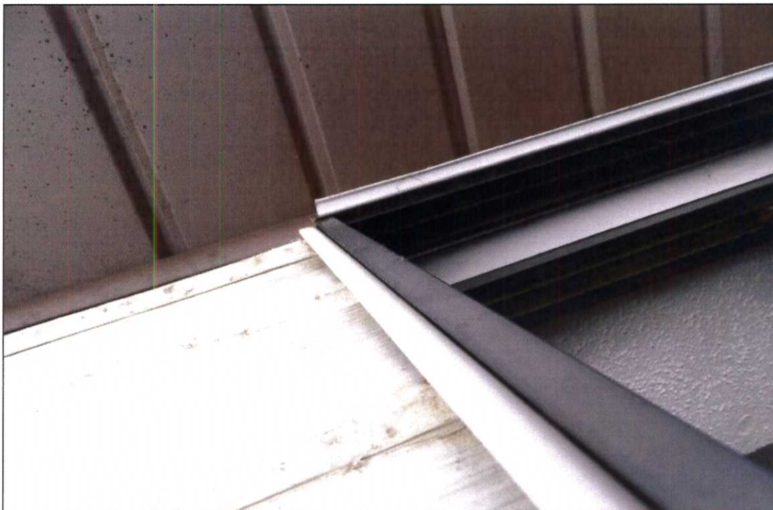
Photograph # 26: No sealant between window frame and vinyl siding.
