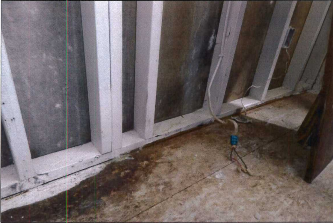
Photograph # 13: Bedroom – water staining on floor; Kilz applied to wall
