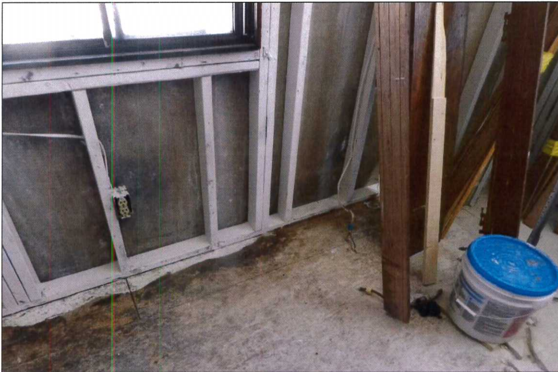
Photograph # 11: Bedroom – water staining on floor; Kilz applied to wall
