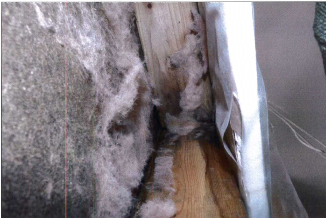
Photograph # 7: Water staining in wall cavity below the window in Photo 4
