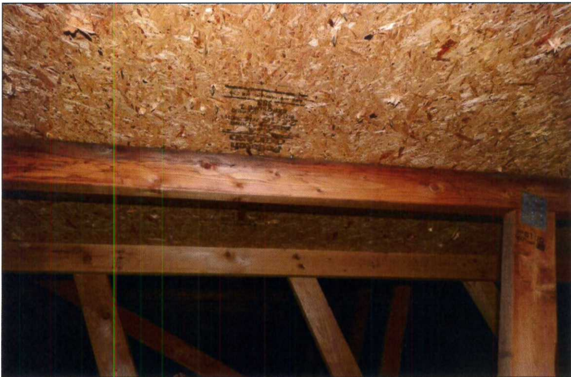
Photograph # 18: minor staining on trusses
