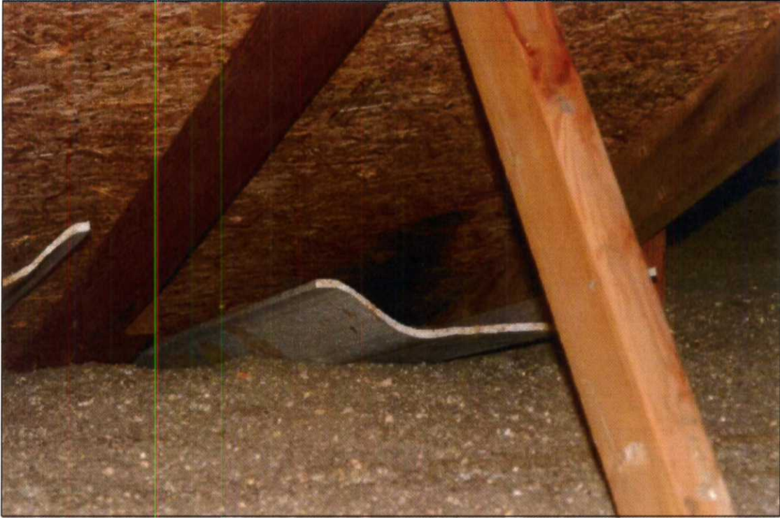
Photograph # 21: Water staining on roof sheathing
