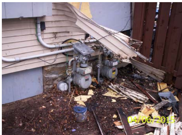
Gas meters locked off
