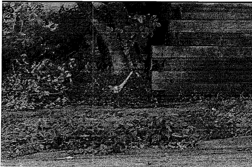
This is the driveway for 778 Jenks, you may be able to tell it extends beyond the east retaining wall approximately 2'
