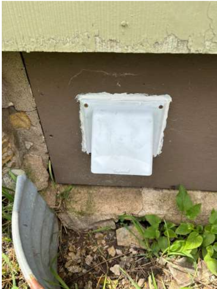
Picture of dryer vent as requested
