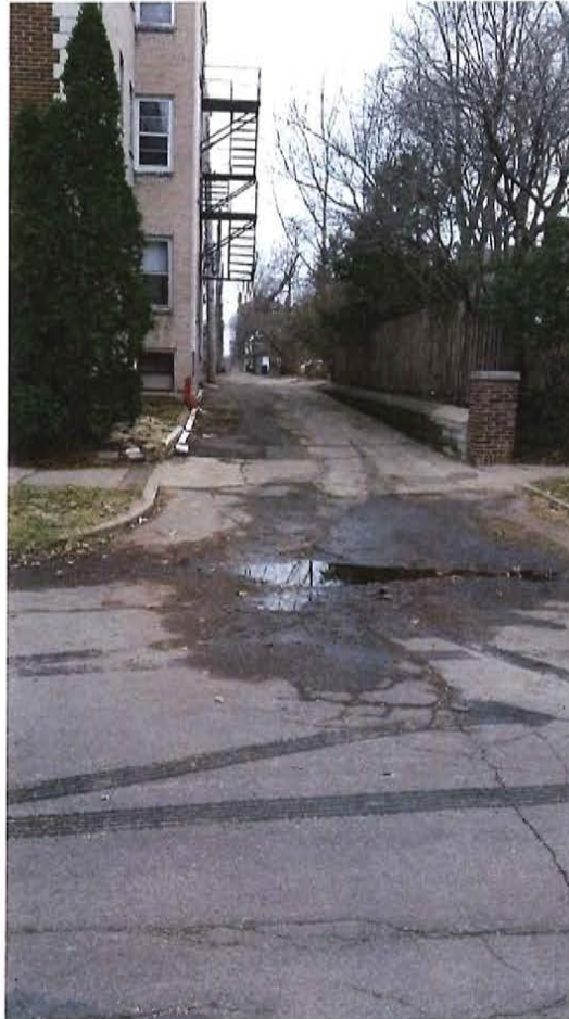
Low Spot in Arundel Street –photo from the Owner dated March 13, 2016
