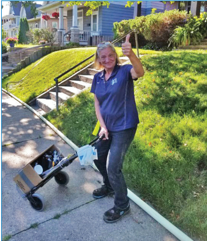
Leeann Smith, water meter tech., works along Selby Ave. where a clean and line project is taking place on the 6-inch and 8-inch pipe. She is installing actuating valves to allow the contractor to backflush the service lines using the temporary water service lines without disruption to the homeowner.
