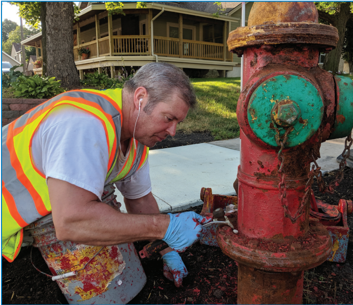
Matt Stone, painter, scrapes a fire hydrant on Aug. 2 at Hoyt and Snelling Ave. to prep it for a fresh coat of paint in time for the Minnesota State Fair, which starts August 22.
