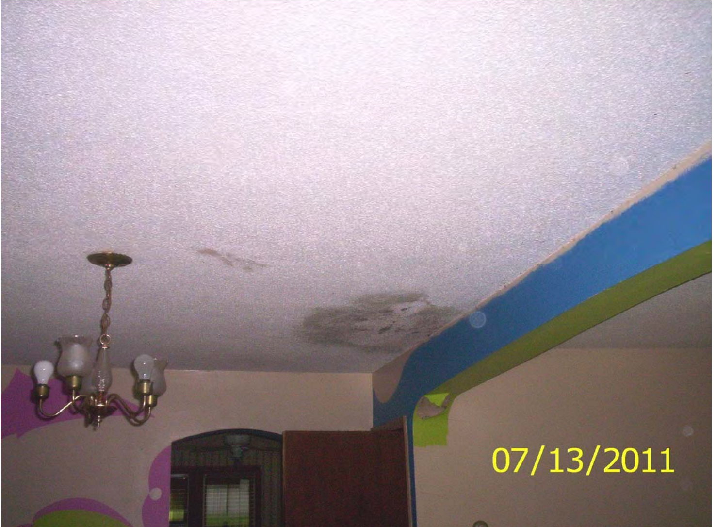
Water damaged ceiling, peeling paint, possibly mold
