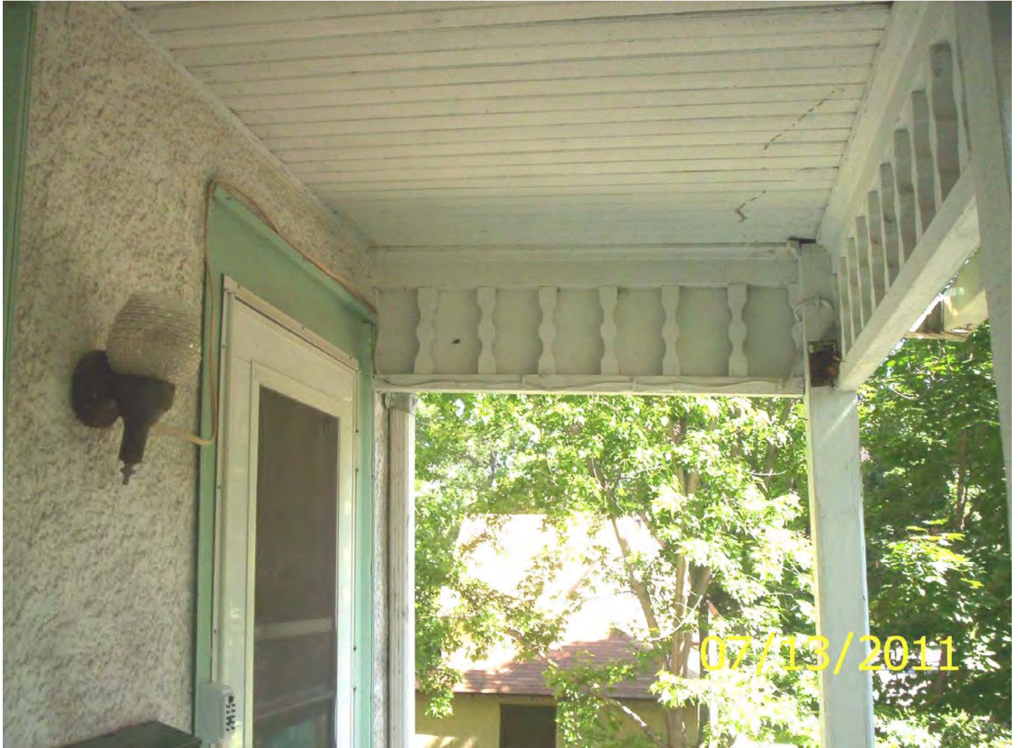
Unapproved exterior electrical wiring
